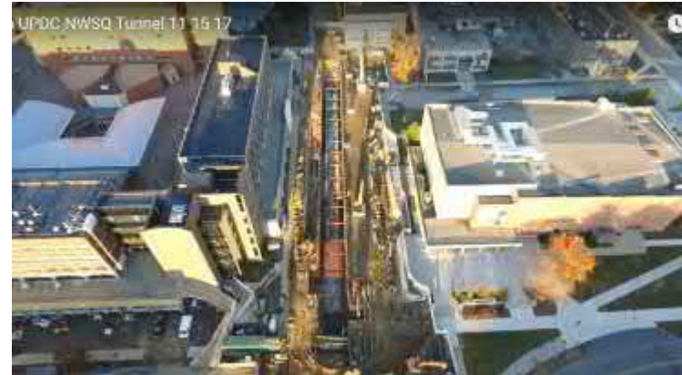
Figure 3.11. Gant Utility Tunnel to the East of the Project Area (November 15, 2017). Source: https://youtu.be/16zqvNcWDAc
