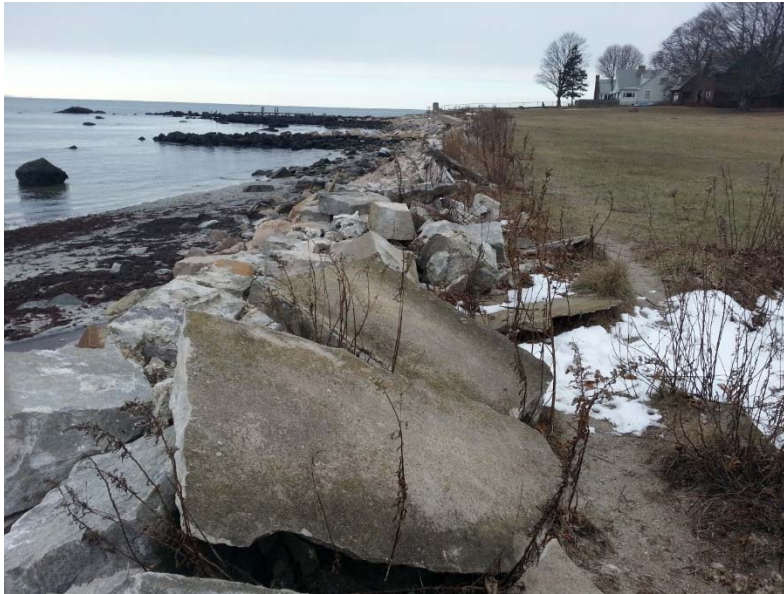
Photo 3-6. Westerly view along broken seawall section
