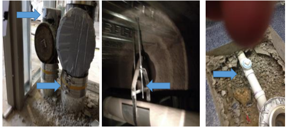
“Plumbing inspection problems”
