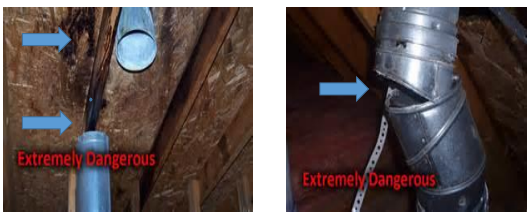
Gas venting "problems"
