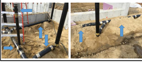
Improper pipe bedding!
