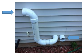
Direct vent termination "problem"
