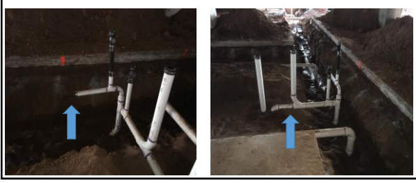
Improperly bedded piping! Should be two stage!
