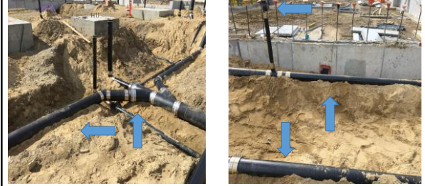
Incorrect pipe bedding.
