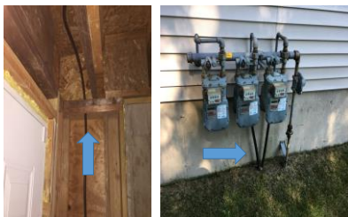
Gas piping issues.
