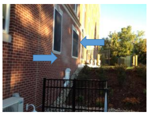
Direct vent boiler termination "problem"
