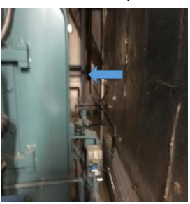
Unacceptable service clearance!
