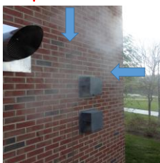
Direct vent intake and exhaust "problem"
