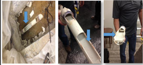
“Plumbing inspection problems”
