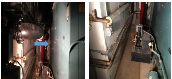
Unacceptable service clearance!
