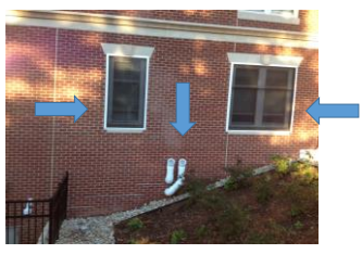
Direct vent boiler termination "problem"
