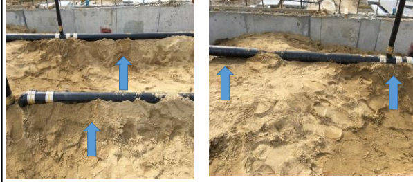
Incorrect pipe bedding.
