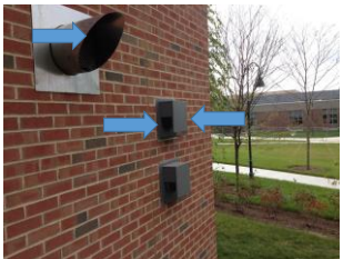
Direct vent intake and exhaust "problem"
