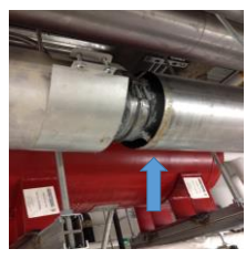
Direct vent gas boiler flue connection
