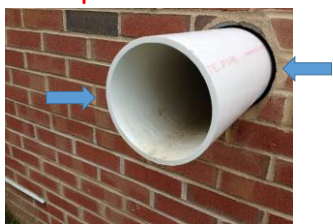
Direct vent water heater termination "problem"
