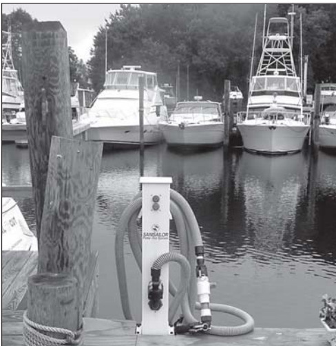
Pumpout station, Brewer Ferry Point Marina, Old Saybrook.
