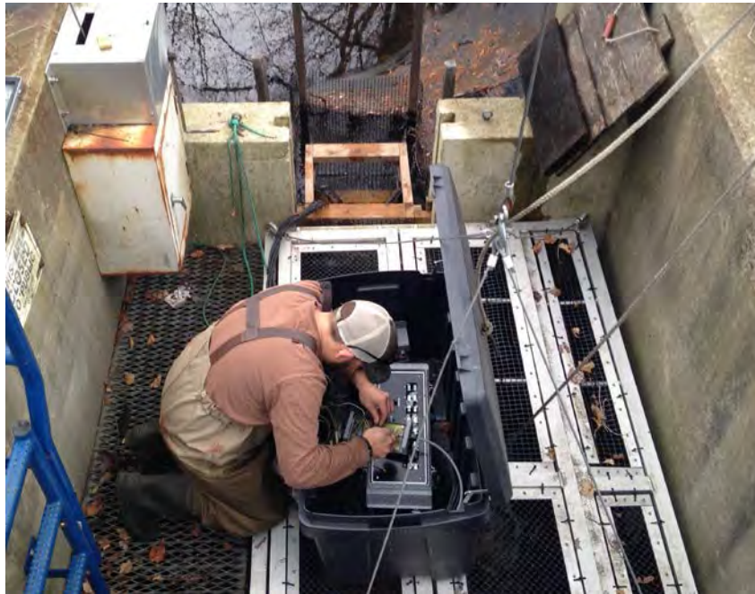
Staff wiring an electronic fish counter at the exit of the Latimer Brook fishway. This counter aids in the enumeration of the Alewife run in this brook.
