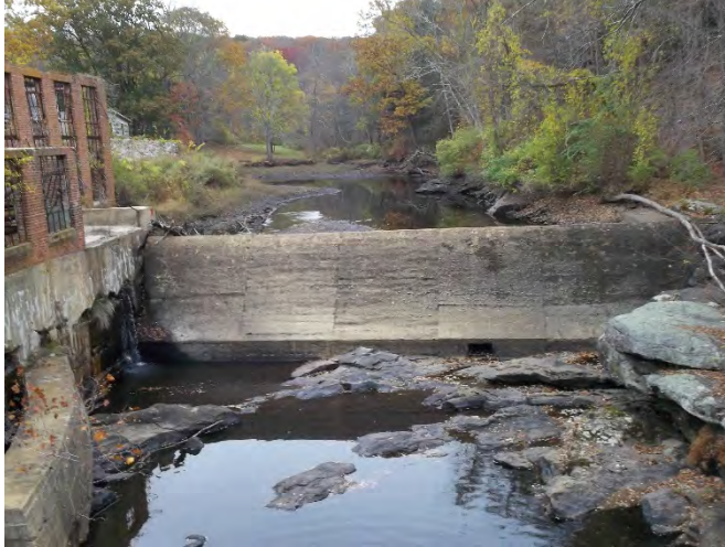
The Norton Mill Dam prior to removal. Note the rock outcrop on the right.
