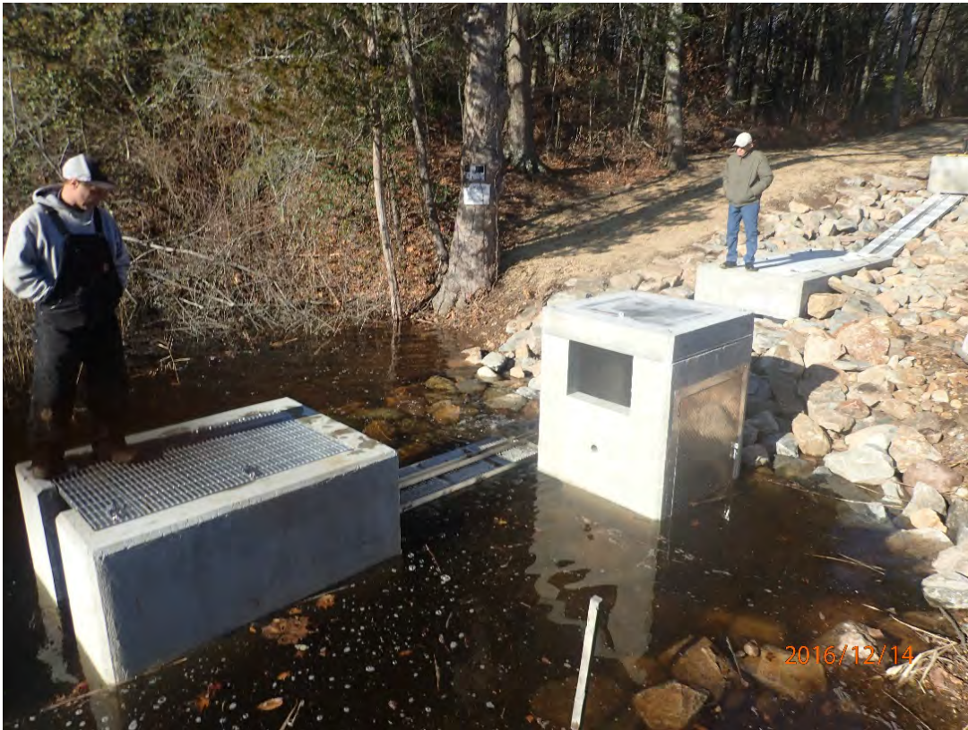
The Chapmans Pond Fishway entrance is back-flooded at extreme high tides. Dave Ellis, to the right, is standing on an intermediate resting pool. Above that, the fishway bends around the corner to enter the headpond through an elaborate trapping and videography station. The large concrete box in the foreground will house an eel pass ramp and trap that had not been installed when this photo was taken.
