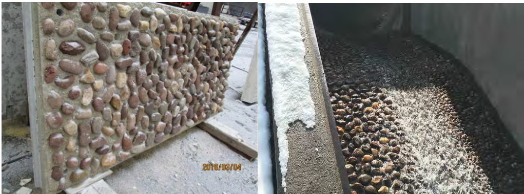
Left- One of the pre-fabricated 9' x 4' concrete substrate panels prior to installation as part of the eel pass. The large gravels will provide passage for large eels. Right- The completed eel pass in the outlet of the perched culvert. Note that the left side panels contain larger gravel than the right side and the water is deeper in the center than along the edges; conditions that provide many passage options for migrating eels.
