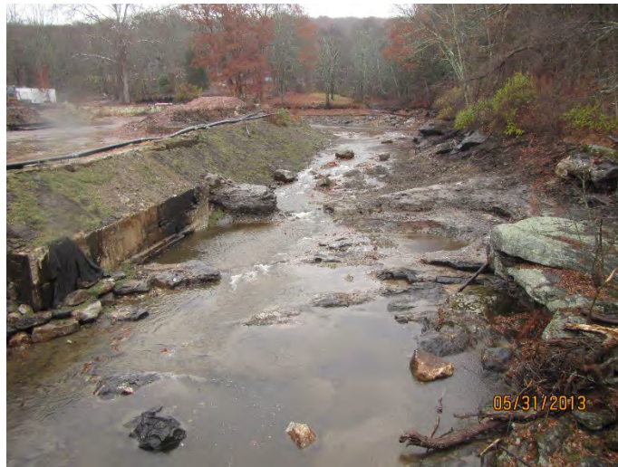
The same view as in the previous photo, after removal. Note rock outcrop.
