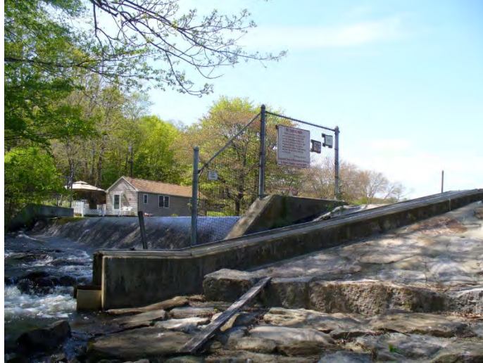
The State-owned Gorton Pond Fishway is located on the Pattagansett River in East Lyme.
