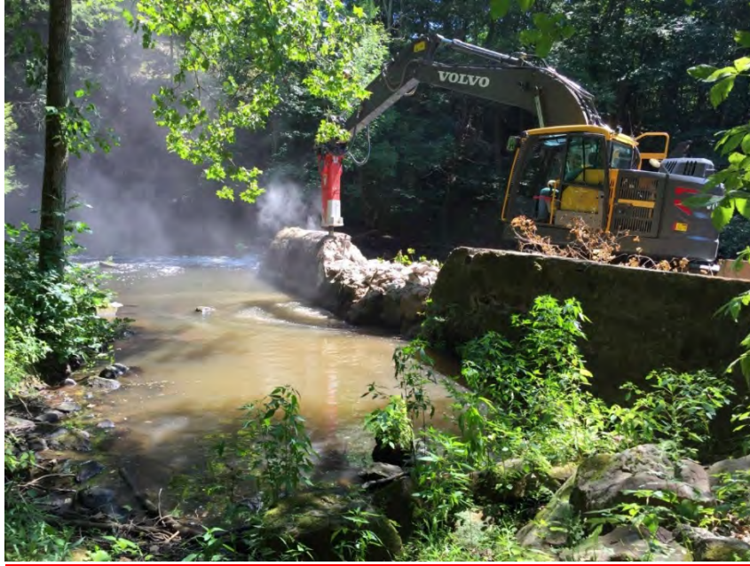
The contractor removing the Carpenters Dam with the use of a 'hoe ram'.
