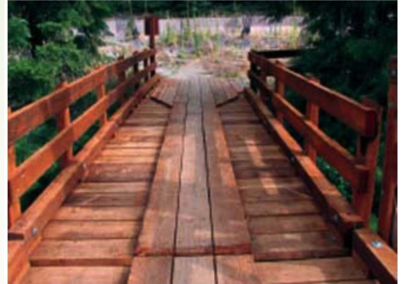
Figure 5-22—Wearing surfaces are a relatively easy and economical way to prolong the life of bridge decking. The tapered pattern guides stock to the wearing surface in the center of the bridge.
