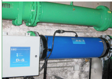
Griswold SBC10000 Reaction Chamber & Control Panel
