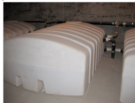
Rainwater Recovery Tanks
