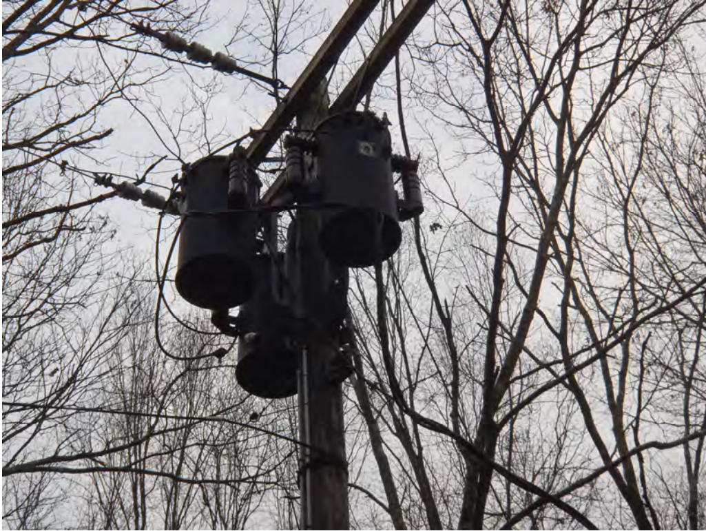
Photo 4-2 – AOC-02 (Pole-Mounted Transformers)
