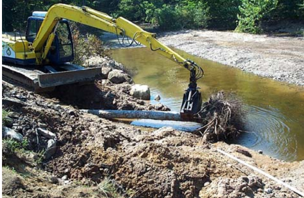
Installation of tree/rootwad complex to provide for erosion control and fish habitat
