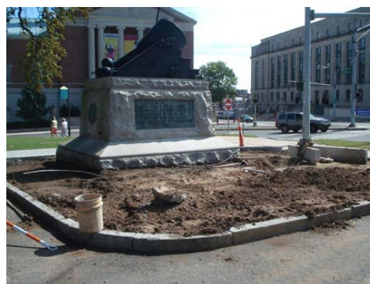
Figure 3.14 – Construction of a rain garden at Hartford Green Capitols Project. Source: Camp Dresser & McKee.
