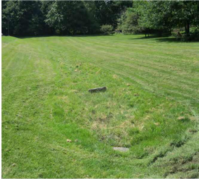
An existing swale identified for potential retrofit to improve stormwater management capability
