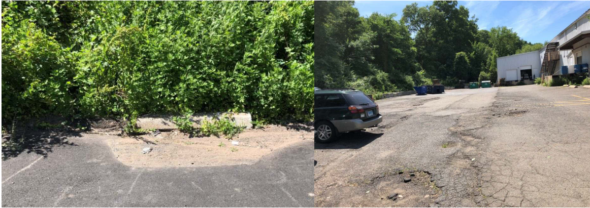
Figure 21. Existing conditions at Counter Weight Brewery, showing clogged catch basin (left) and degraded asphalt parking lot (right).
