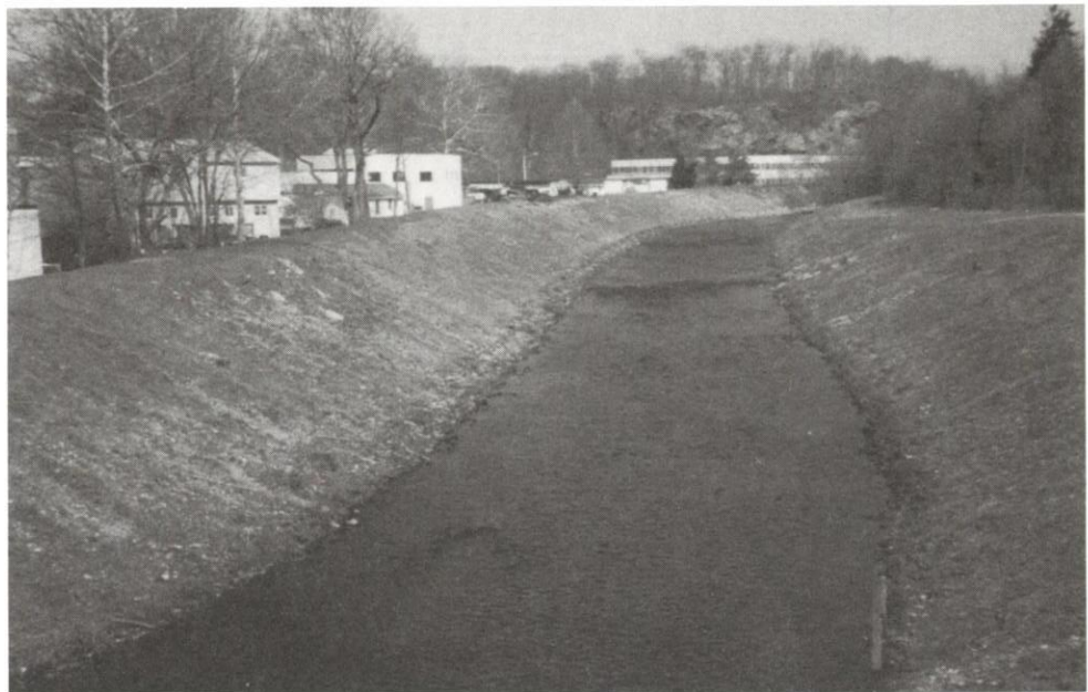
Photo: A channeled section of the Norwalk River provided for flood relief but provides few, if any, water quality or habitat benefits.
