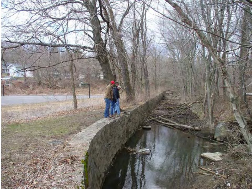
Figure 12: Historic rock channel and side wall. (Photo courtesy of Carol Donzella, NRCS Community Planner)
