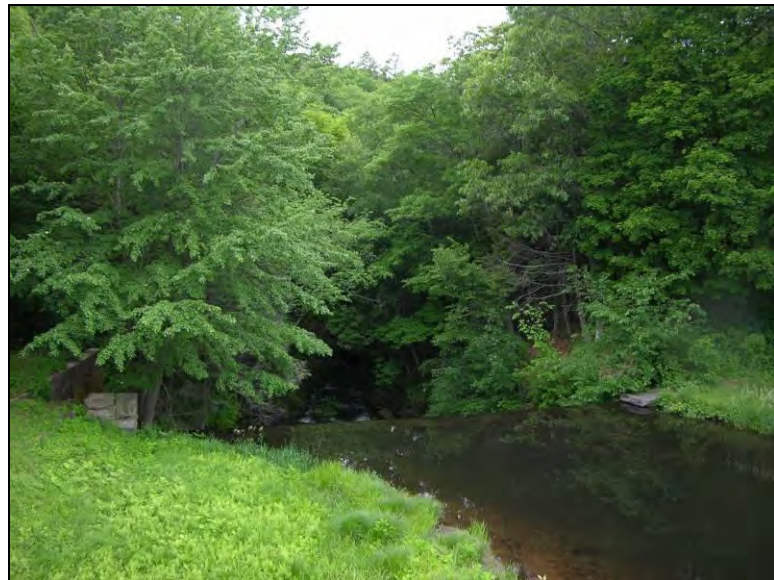
The upstream side of Dobsonville Pond dam at the upstream limit of reach LTR-03. The photograph is taken near the confluence with reach TB-01.
