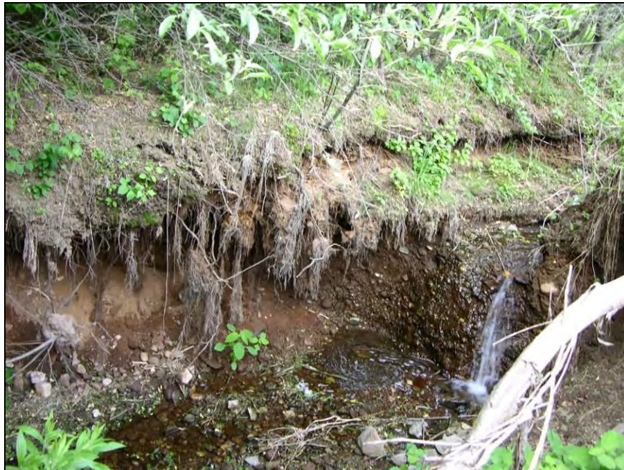
Eroded channel and discharge from a residential property.
