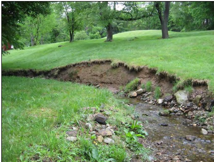
Stream segment GB-05B showing area of stream bank erosion.
