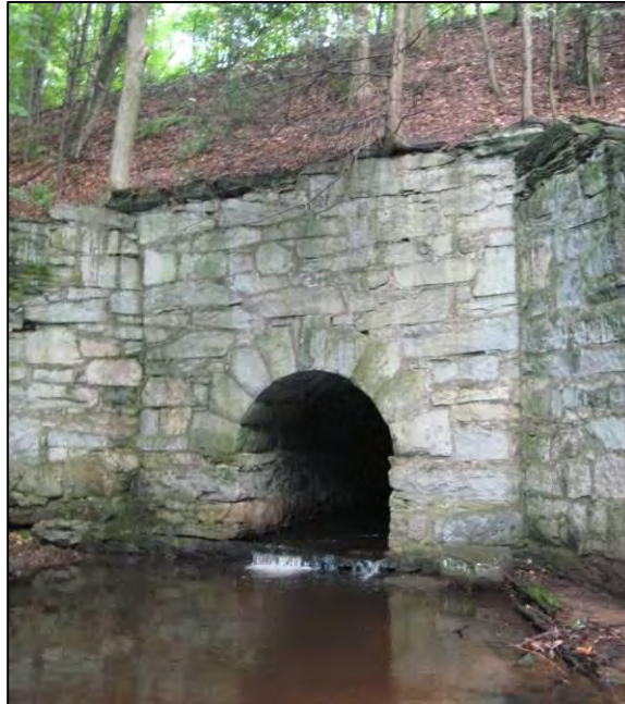
Arch-type railroad crossing (SC-02) constructed of stone and extending approximately 125 feet. The crossing may prevent fish passage and is suffering from downstream scour evidenced by the large pool shown in the photograph.
