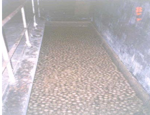
Grease buildup at a wastewater pumping station
