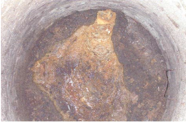
Grease buildup obstructing a sewer manhole
