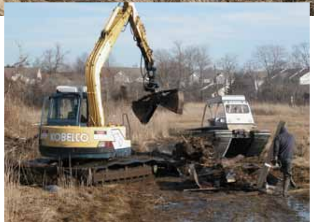
Using a clamshell bucket, the low ground pressure excavator loads debris into the sled.
