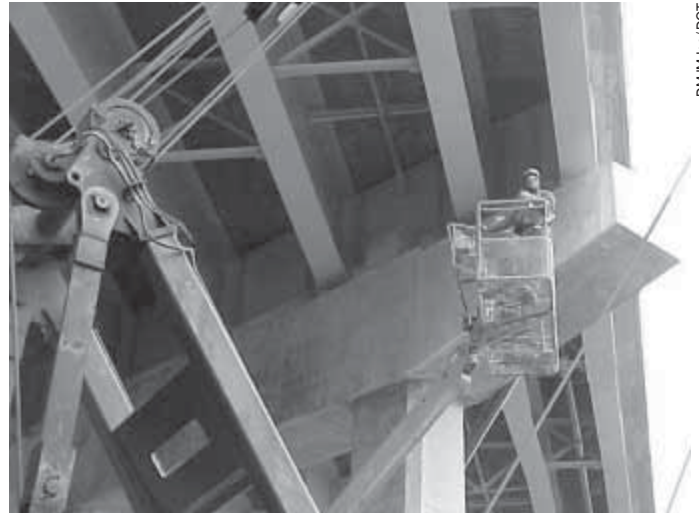
Contractors for the DOT finish installing one of three peregrine falcon nest boxes on the P. T. Barnum Bridge in Bridgeport.
