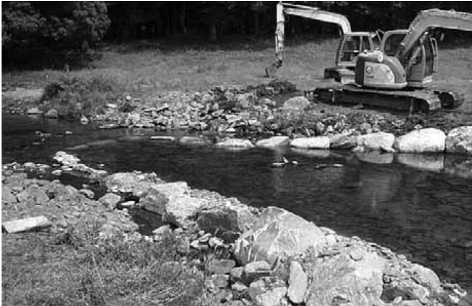
Completed construction of a cross-vane rock structure (note upstream horseshoe shape) designed to deflect flow away from streambanks.
