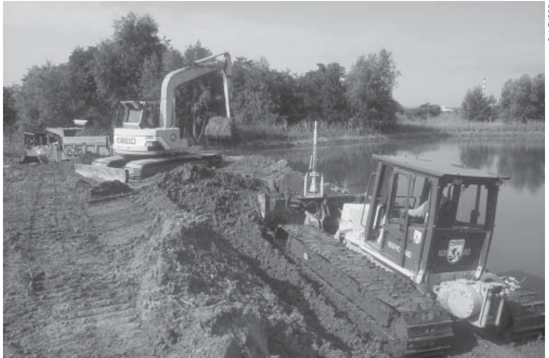
At a restoration site in Stratford, the WHAMM crew uses a bulldozer and excavator to remove spoil material that is loaded into a dump truck. Approximately 35,000 cubic yards of fill are slated to be removed to restore the marsh to the proper elevation.
