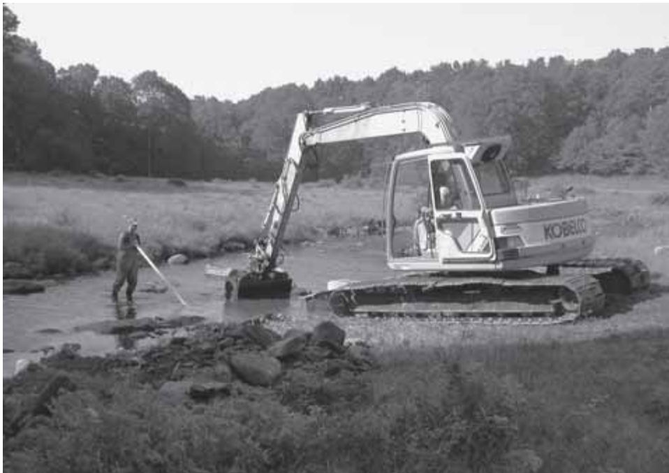
Donald Hargreaves, of the WHAMM Program, operates a specialized excavator along the Mount Hope River in Ashford, while Brian Murphy, of the DEP Fisheries Division, uses a stadia rod to determine the rock depth for a cattle crossing.
