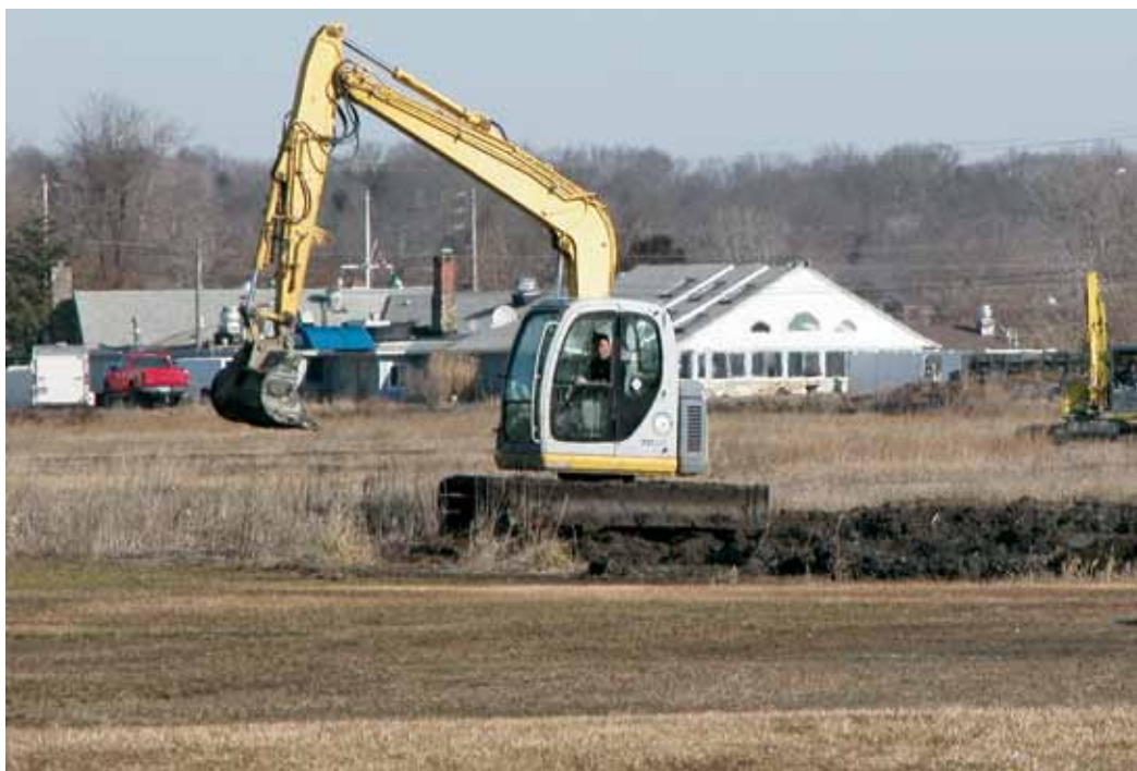
A low-ground pressure excavator is used to create a new pool and clean old mosquito control ditches in the Jacob's Beach Marsh in Guilford.
