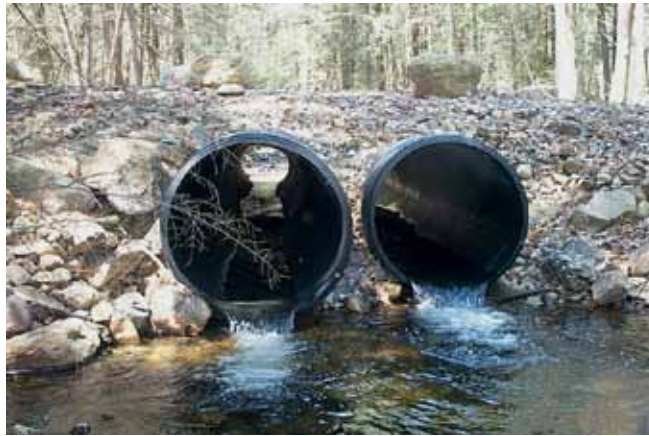
Before restoration: Perched twin culverts at a stream crossing of Leadmine Brook, in Ashford, blocking upstream fish passage for native brook trout.
