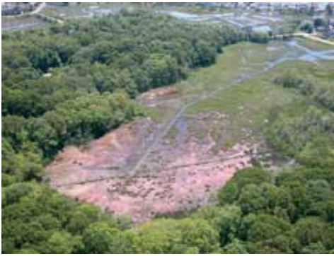
A view of the wetland restoration work conducted at Groton Long Point. A long channel was excavated to allow tidal water in and out of the site. This photograph was taken on June 8, 2012.
