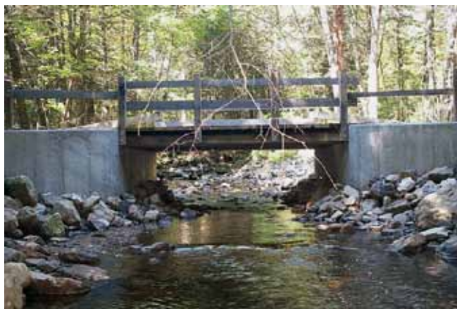
After restoration: Leadmine Brook twin culverts were removed and replaced with a clear span timber bridge, thus restoring fish passage to 2.9 miles of upstream habitats.
