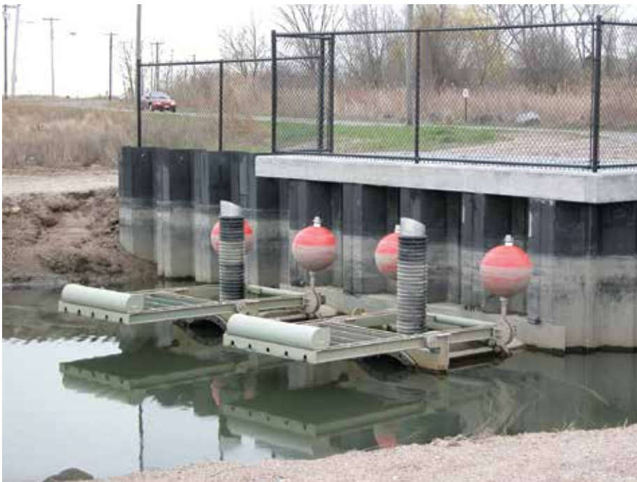
Self-regulating tide gates (SRTs) increase tidal flow without causing upstream flooding.
