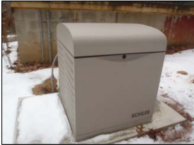
North Willington Village Emergency Generator Funded by Emergency Power Generator Program Administered by DPH
