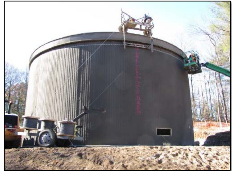
Tarriffville Fire District New Storage Tank Funded by Drinking Water State Revolving Fund Administered by DPH
