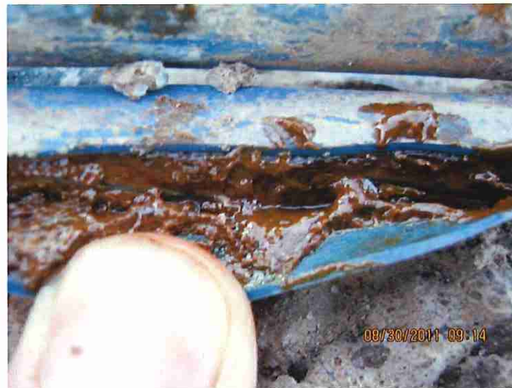
Figure 6. Emulsified grease on post-tensioning grease.
