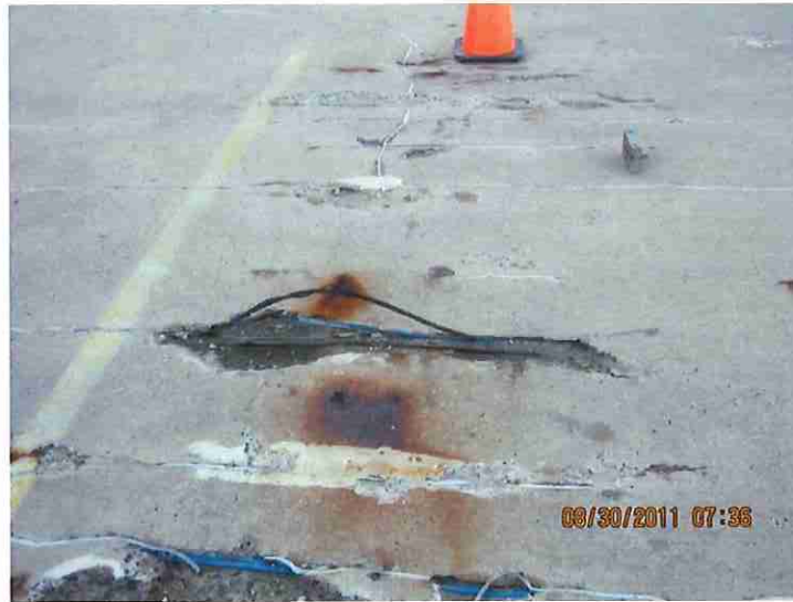
Figure 5. Failed post-tensioning on Level 6.
