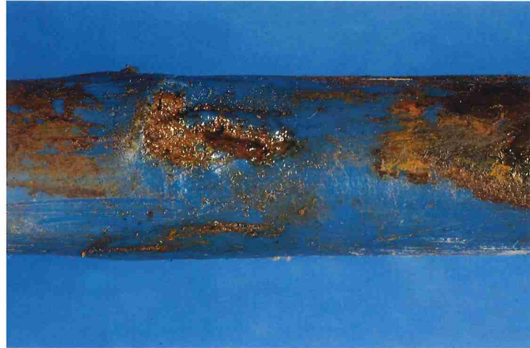
Figure 3. Second location of many on strand #1 showing evidence of sheath damage.
