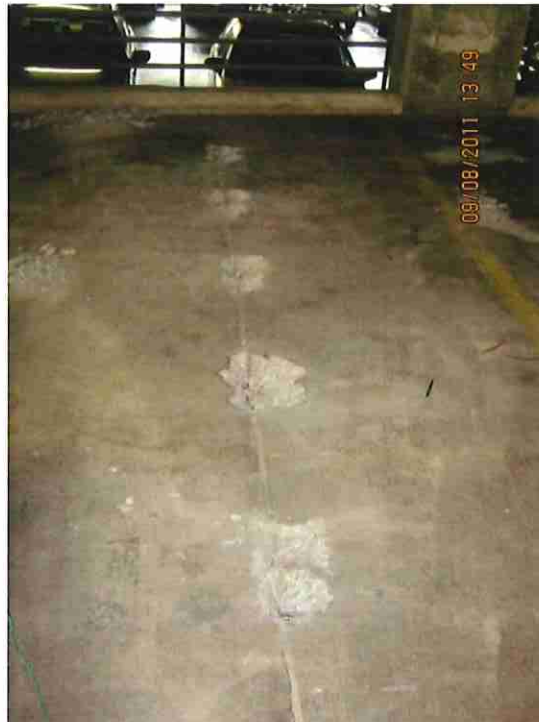
Figure 9. Openings at construction joint on Level 2.
