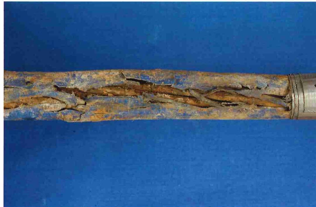
Figure 4. Severely damaged PE sheathing and visibly corroded strand wire on strand #2. L3607 093011 04
