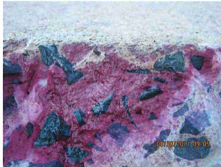
Figure 16. Concrete surface on Level 6 with phenolphthalein applied.
