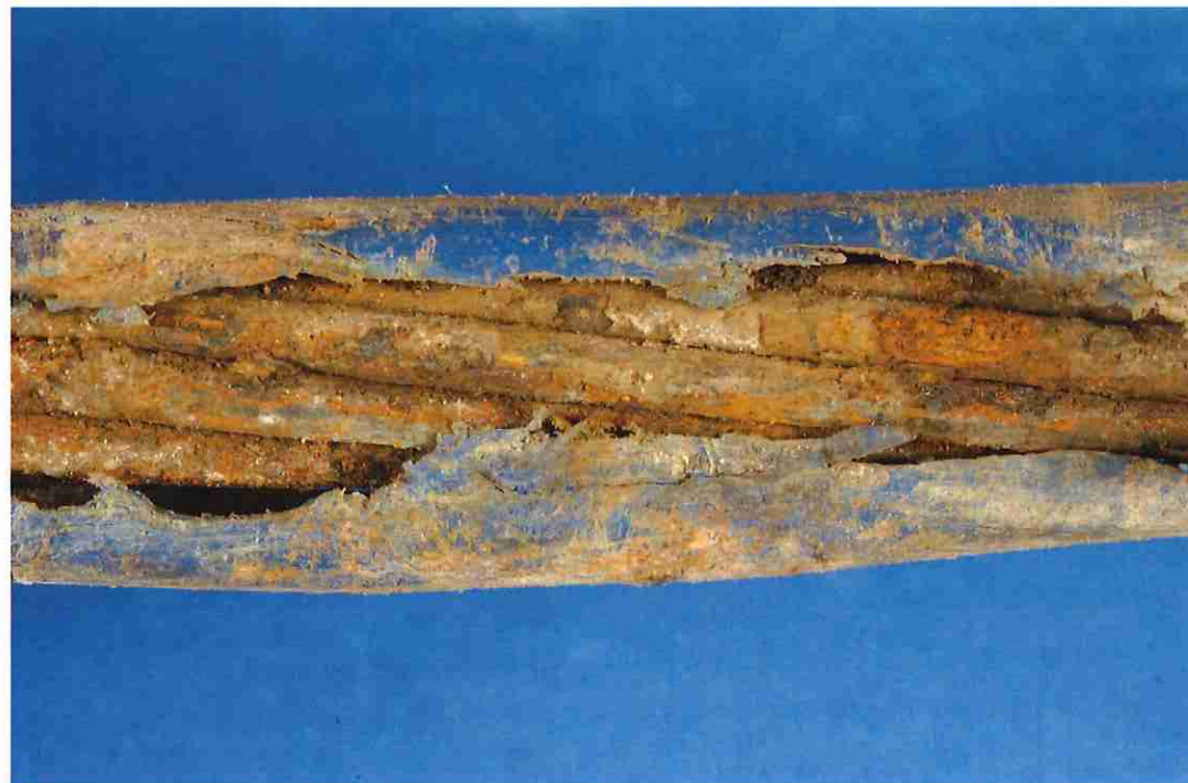
Figure 6. Second location of sheath damage and strand wire corrosion on strand #2.
