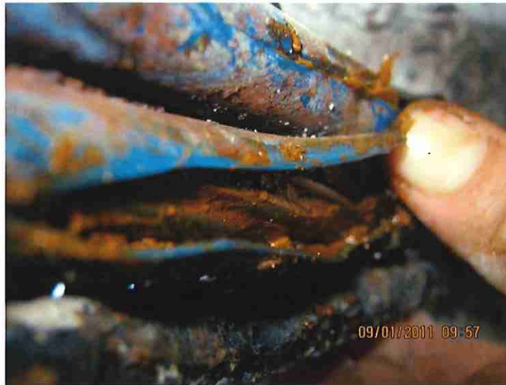
Figure 14. Water and emulsified grease on strand.
