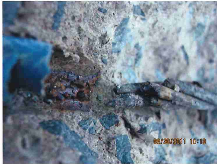
Figure 7. Brittle failure of post-tensioning strand on Level 6.
