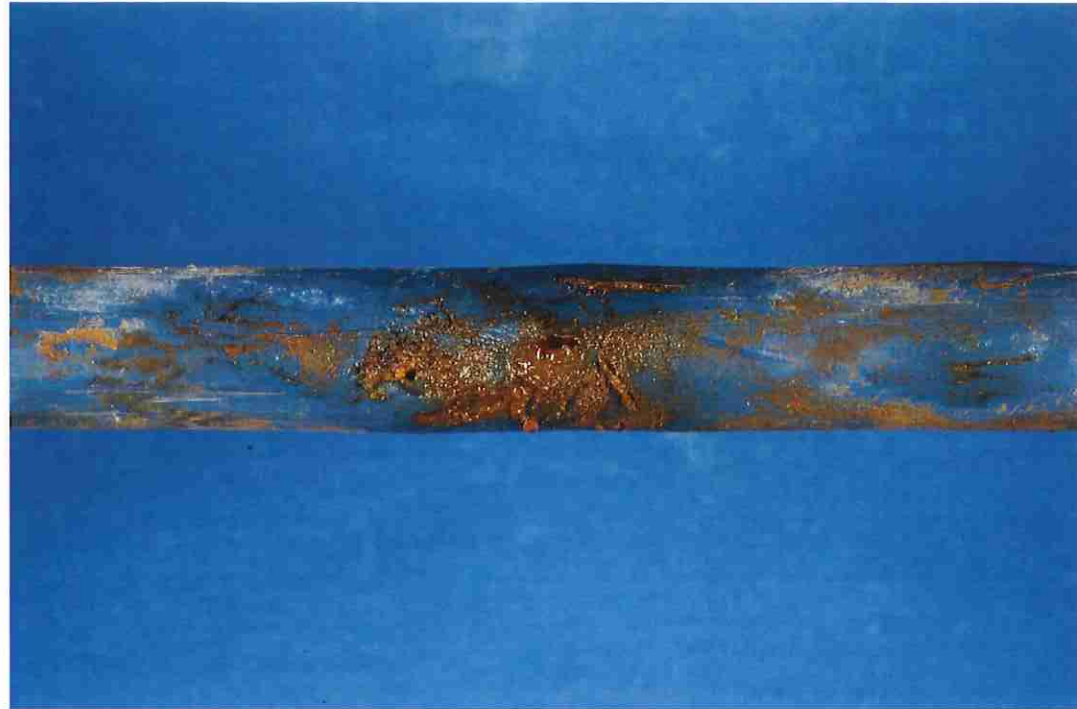
Figure 1. View of a portion of strand #1 identified as “L6 South E Centerline” at a location of damage to the polyethylene (PE) sheath where iron corrosion product stained grease is visible. L3607 093011 01
