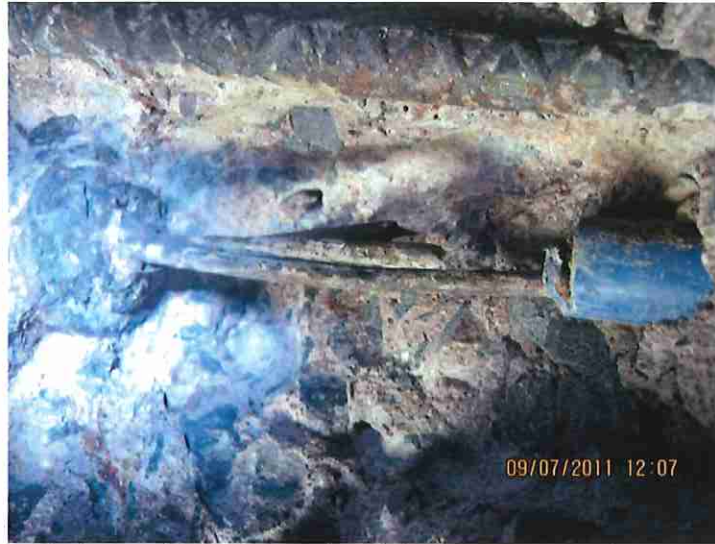
Figure 10. Failed strand at construction joint. Note corrosion on anchorage and failed wires.
