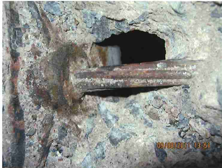
Figure 11. Corrosion damage on strand, without strand failure.
