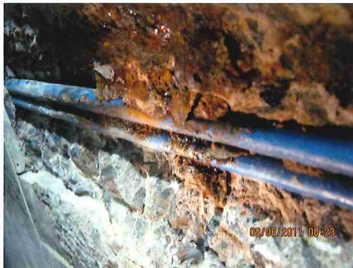
Figure 15. Corrosion damage to mild reinforcing steel and damage to sheathing on soffit.
