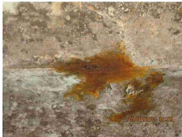
Figure 13. Water dripping through construction joint in vicinity of failed strands.
