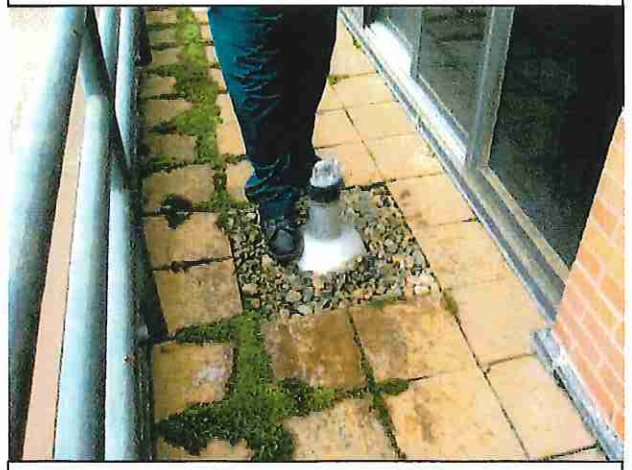
Moss growth / Water Infiltrating scaffolding Anchor Points
