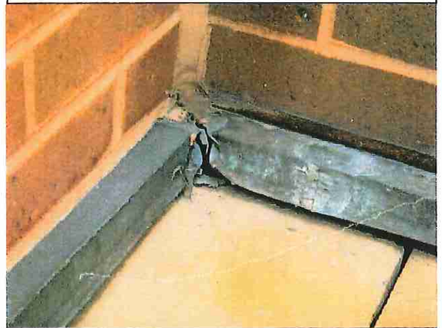
Excessive Sealant and Damaged Flashing
