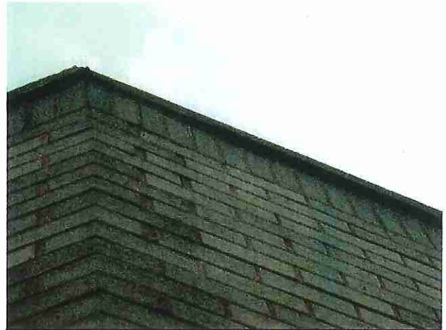
Failing Mortar Joints
