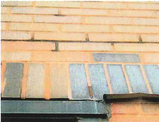
Moisture trapped in wall not coming out weeps
