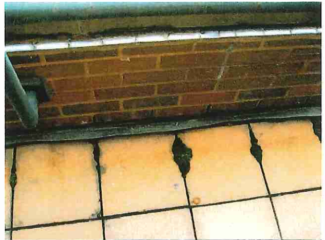
Damaged Thru-Wall Flashing (typical)
