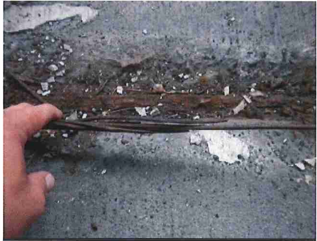
Photo 6 Broken P/T Cable at floor spall.
