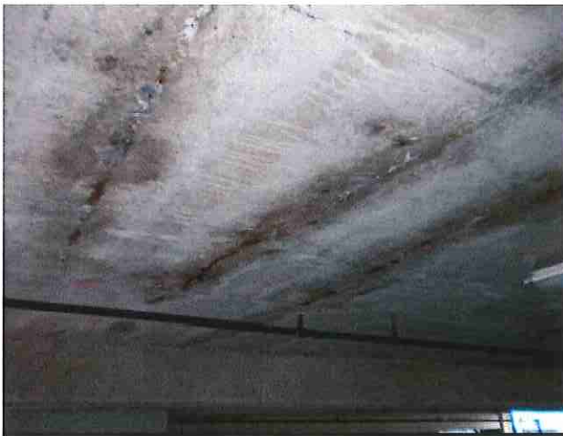
Photo 3 Typical cracking in P/T slab viewed from the underside.
