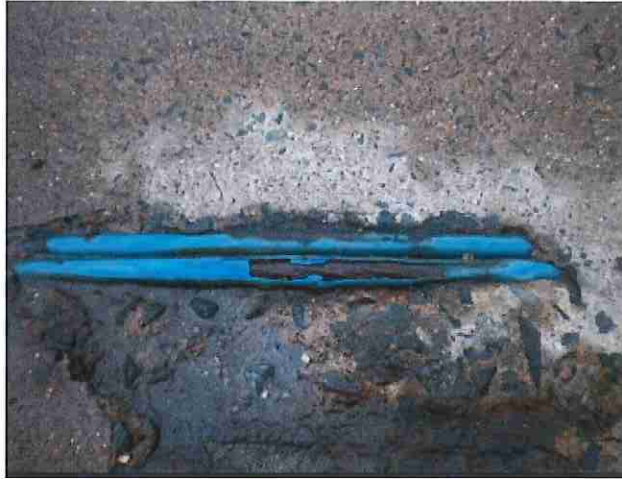
Photo 5 Exposed P/T cables on the Roof Level with damaged sheathing.
