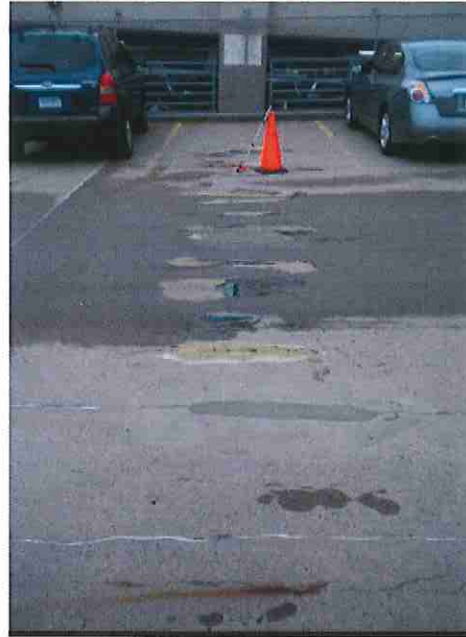
Photo 2 Typical slab deterioration over concrete beams.
