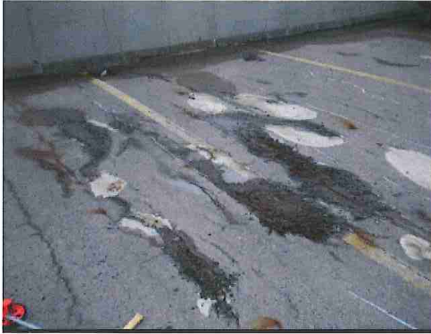
Photo 1 Typical slab deterioration on the Roof Level
