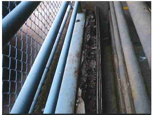
Photo 16 Slab deterioration at pedestrian guardrail.
