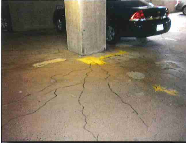
Photo 9 Typical sealed cracks in the East Side floor slabs.
