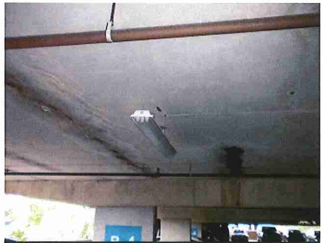
Photo 4 Typical cracking in P/T slab near cantilevered end of beam.
