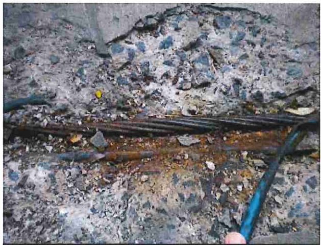
Photo 8 Exposed P/T cable with apparent separation of strands, indicative of a possible break.
