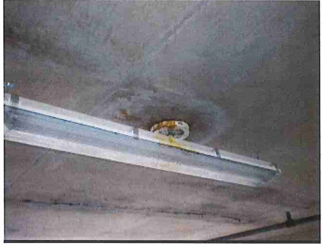
Photo 18 Leakage and rust staining at light fixture.
