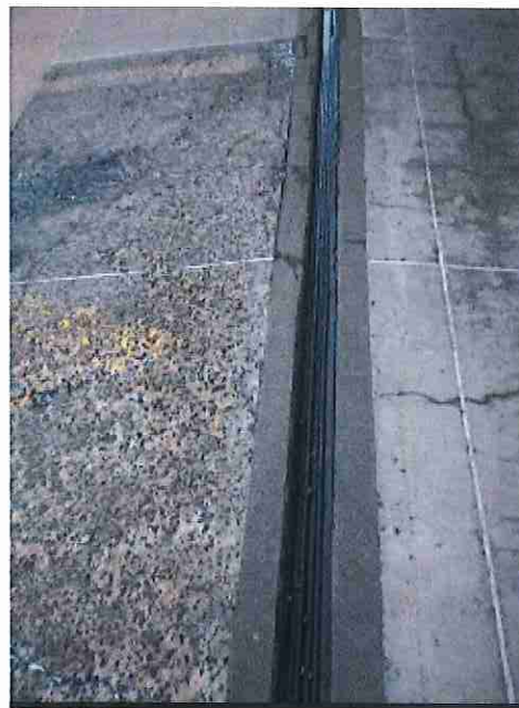
Photo 12 Roof Level expansion joint. Note scaling of concrete wash.
