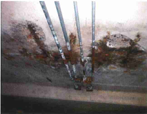
Photo 11 Spalling on the slab beneath the garage exit.
