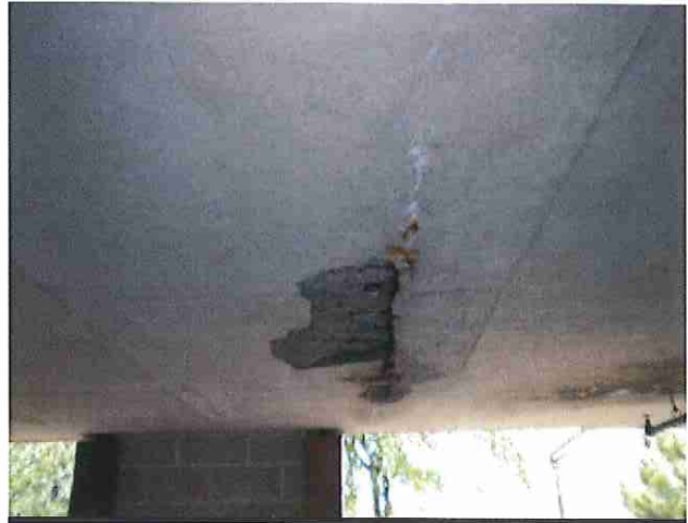
Photo 10 Spalling on the underside of the East Side Slab.
