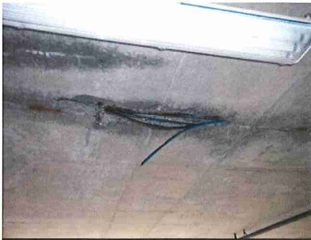
Photo 7 Broken P/T cable that has burst through the bottom of Level P-3 Slab.
