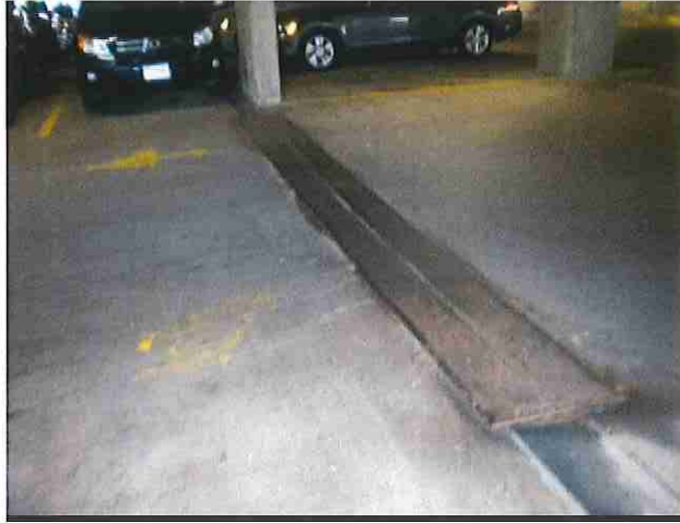
Photo 13 Typical condition of expansion joint between the East and West side. Note steel cover plate.
