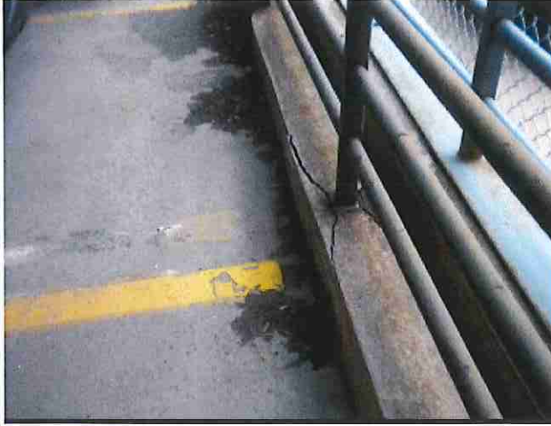
Photo 17 Curb deterioration at pedestrian guardrail.
