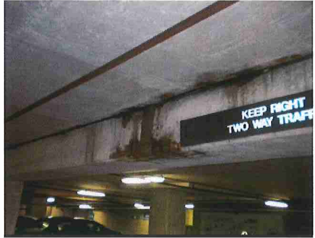
Photo 14 Leakage on beam below the expansion joint.
