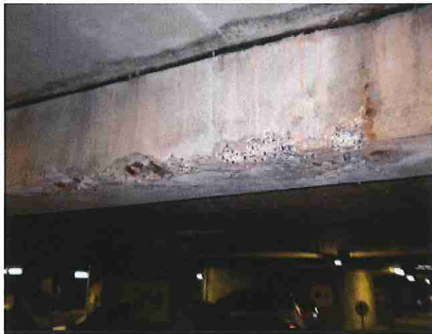
Photo 15 Spalling of concrete beam below expansion joint.
