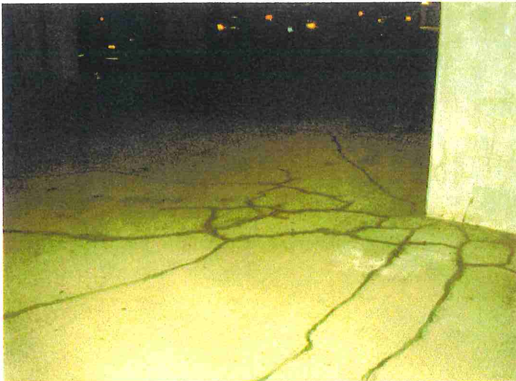
Photo 11 - Typical cracking around columns east of column line "K" in two-way slab negative moment region. Crack seals need repair.
