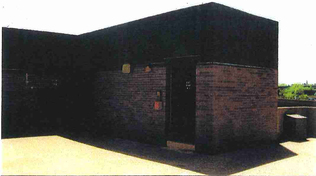
Photo 26 Temporary repairs made to southwest stair core. Needs proper reconstruction
