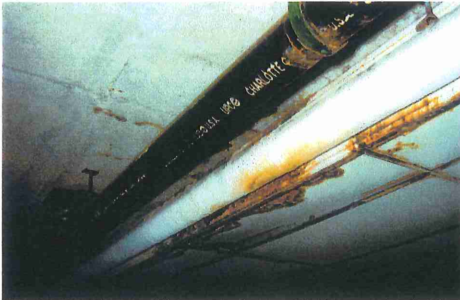
Photo 7: More evidence of soffit deterioration.
