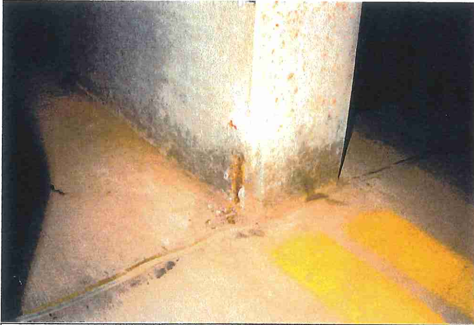
Photo 21: Spalling over column bars has occurred in several places at the floor level. Minimum cover was not provided; repair required.
