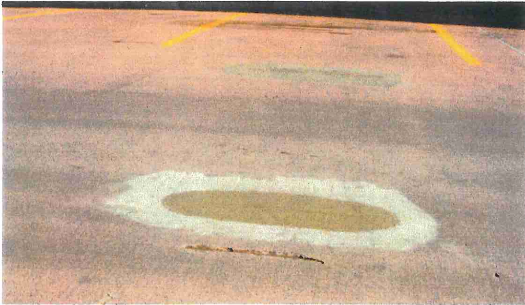
Photo 19 Previous epoxy type repairs in roof deck and exposed embedded rebar in foreground needing similar repair
