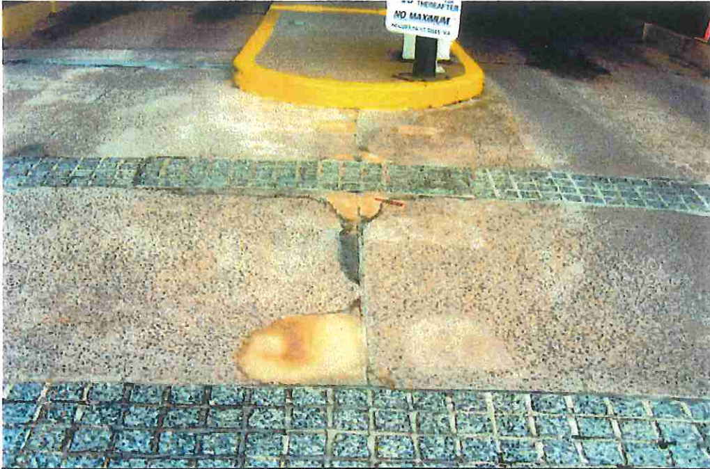
Photo 3: Previous repairs at entrance. Area needs reconstruction to protect structure below.
