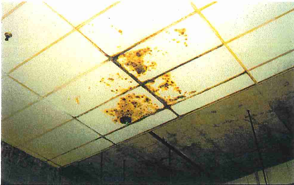
Photo 6: Moisture affects 12" plaza slab, ceiling elements below (P3 level soffit shown here ) and any embedded mechanical systems (including slab heating grid)
