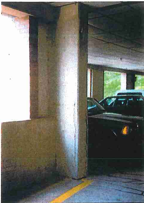
Photo 8: Column near entrance at Column Line intersection "N-12". Two vertical bars (at corners) are bowing out approx. two feet above floor. See photo #10.
