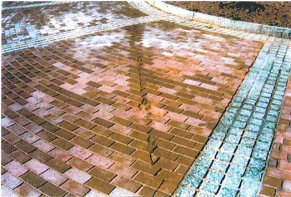
Photo4: Garage extends under the plaza area up to this crack (garage is to the right of the line).
