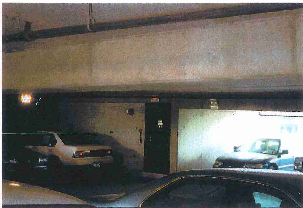
Photo 28 In some areas the sight lines to exit signs are obstructed.
