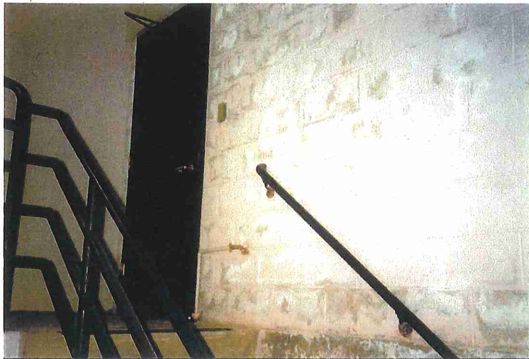
Photo 27 Efflorescence on inside wall of staircore.
