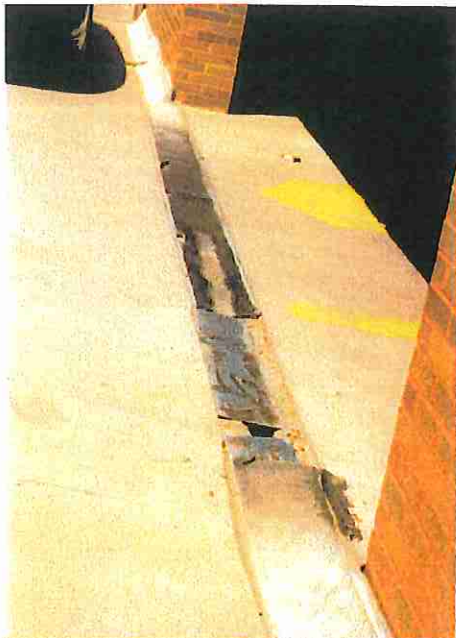
Photo 13 - Expansion joint at roof looking north along column line "K". Joint is damaged and is leaking along entire length. Joints at all levels should be replaced.
