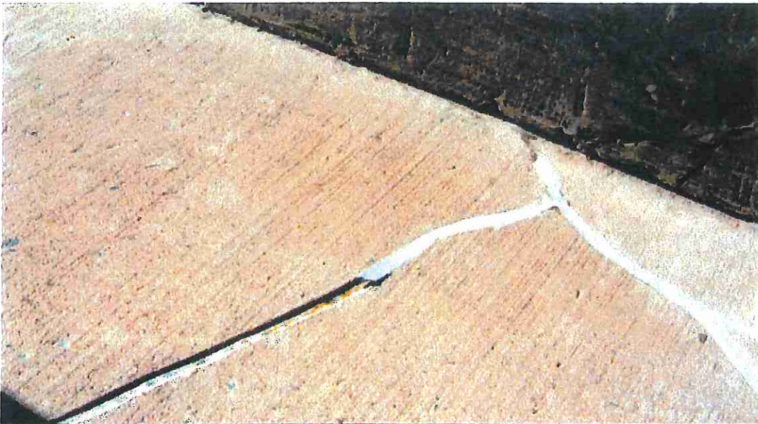
Photo 20 Crack sealant is aging and failing. Note no cove joint at parapet; should install new cove joints.
