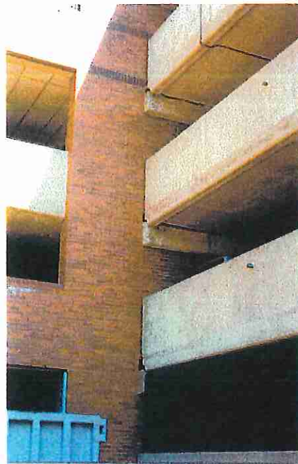
Photo 14 - Expansion movements and leaking joints have caused cracking at support ledge at "K-8". Neoprene bearings on ledge absorb expansions.
