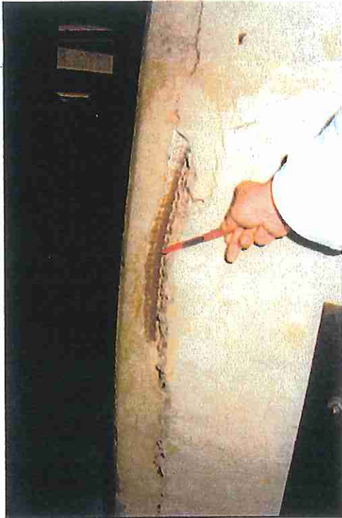
Photo 10 - Bar bowing. Indications are that the rectangular horizontal tie at this one elevation does not wrap outer two corner bars.
