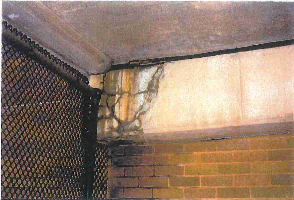
Photo 15 Close-up of typical damage at locations observed in photo 14. Bottom corner of parapet (above fence post) should be chipped back where it is touching ledge support. Note black neoprene bearing disappearing behind this parapet lip.
