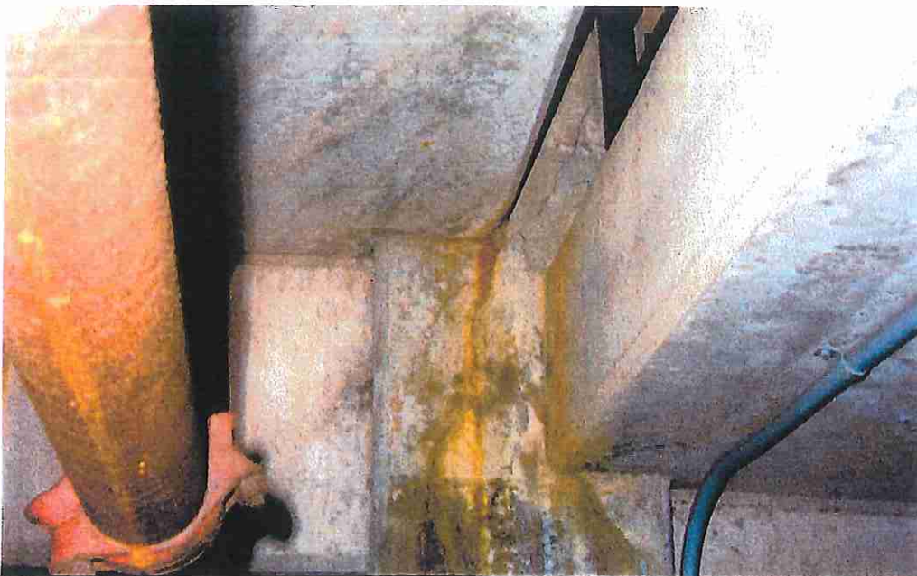
Photo 24: At column line 5, where ramping bay beams connect to columns some cracking is occurring. Note evidence of heavy moisture and that column is loaded asymmetrically at two different elevations (sloping ramp configuration)
