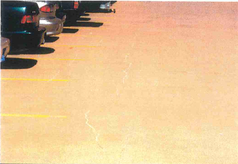
Photo17 - Cracks with white sealant at roof slab run tranverse to axis of cantilever beams (cantilevered section is under cars). PT running in the direction of the cracks cannot prevent them. Tension in this negative moment region tends to open these cracks as the slab acts compositely with the cast-in-place cantilever beams.
