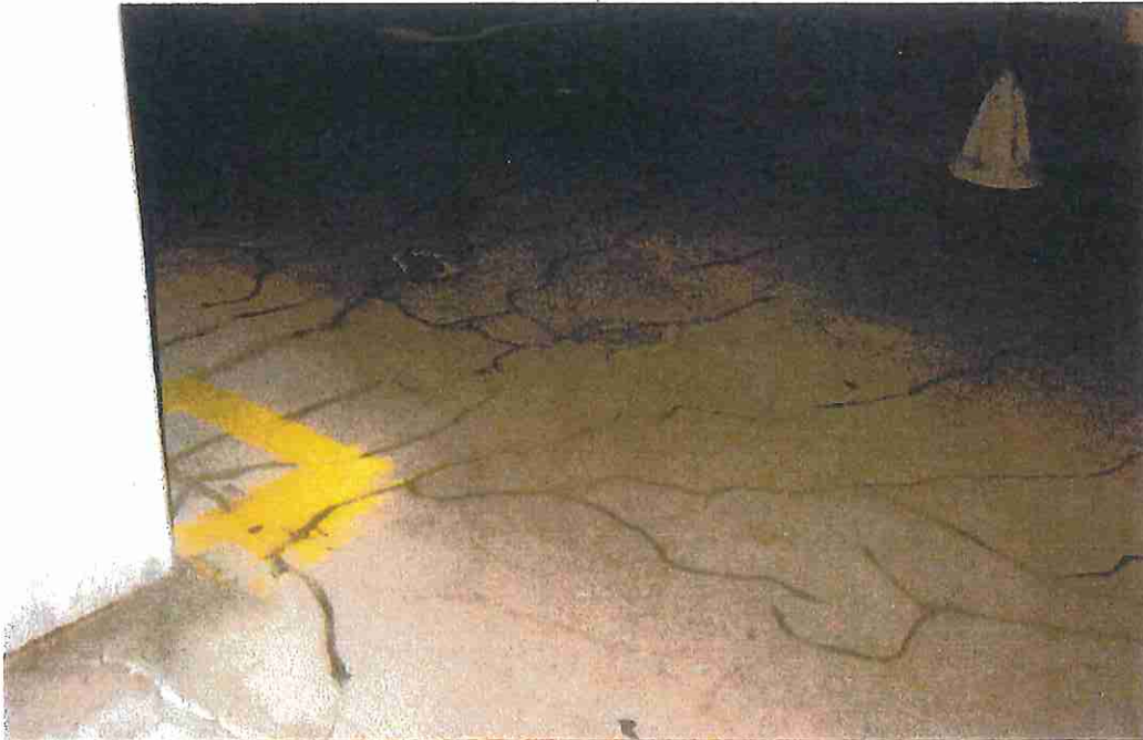
Photo 12 Another example of two-way slab cracking at tower building garage. Note new cracks that need routing and sealing to protect tension reinforcing below.
