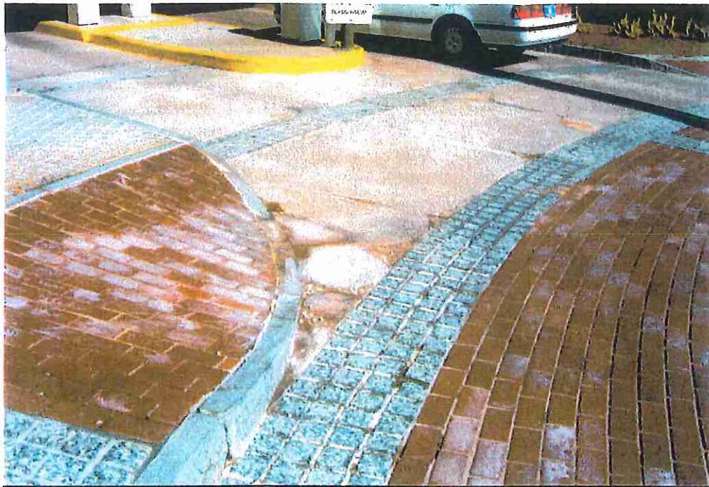
Photo 2: Entrance surface of brick, stone and concrete is deteriorating. Moisture and chlorides are penetrating through to structural elements as shown in photos to follow .
