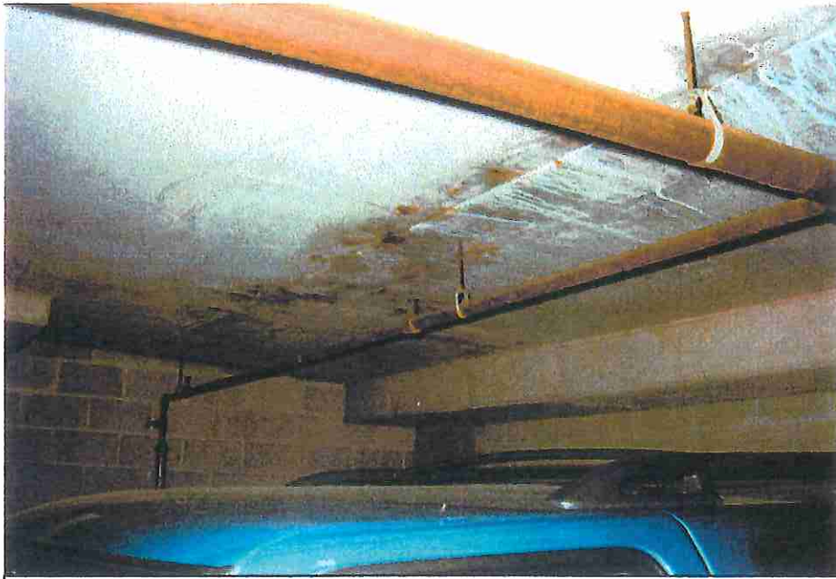
Photo 5: Result of moisture penetration from entrance above; chloride deposits and ongoing corrosion.
