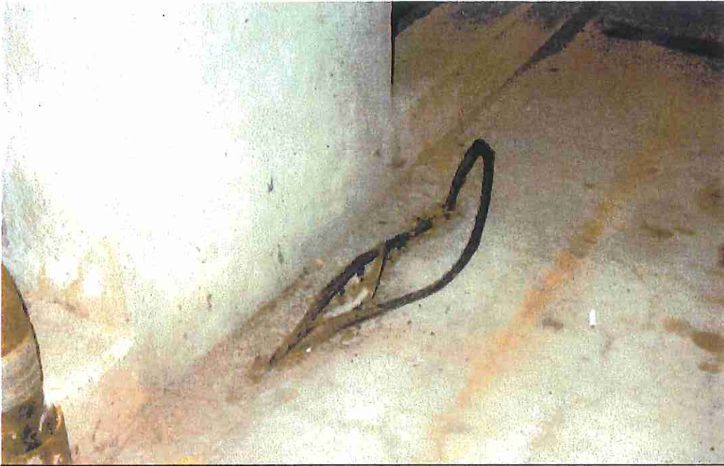
Photo 29 One post-tensioned strand was found “popped”. Due to the location this is not a concern. It is an example, however, of what could happen if proper repair and maintenance is not preformed.
