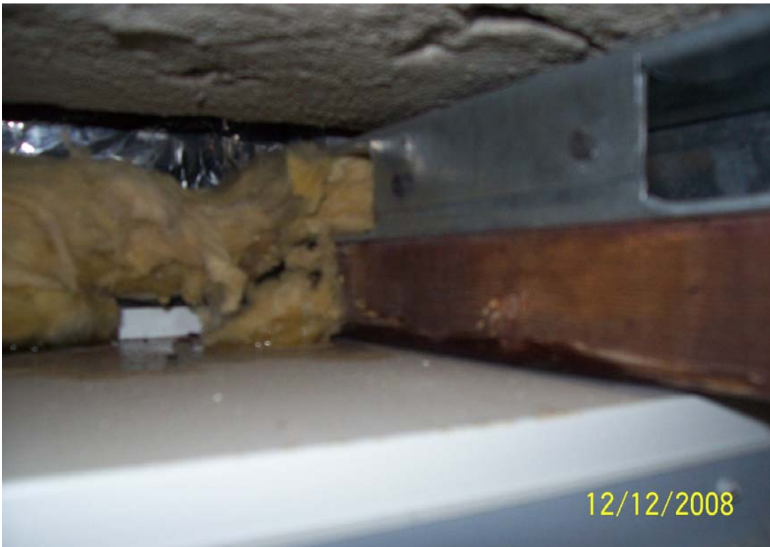
Water Observed Infiltrating the Window Head on the 17 th Floor
