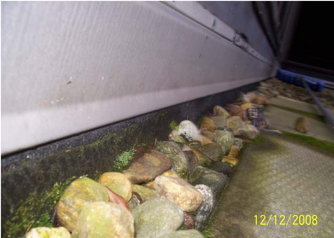
Moss Growing on Roofing Member below Window Sill on 7 th Floor Roof (Located directly above leak on 6 th Floor)
