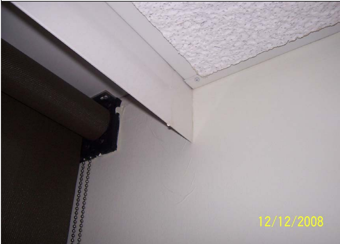
Small Drip of Water in Corner of Window on the 17 th Floor
