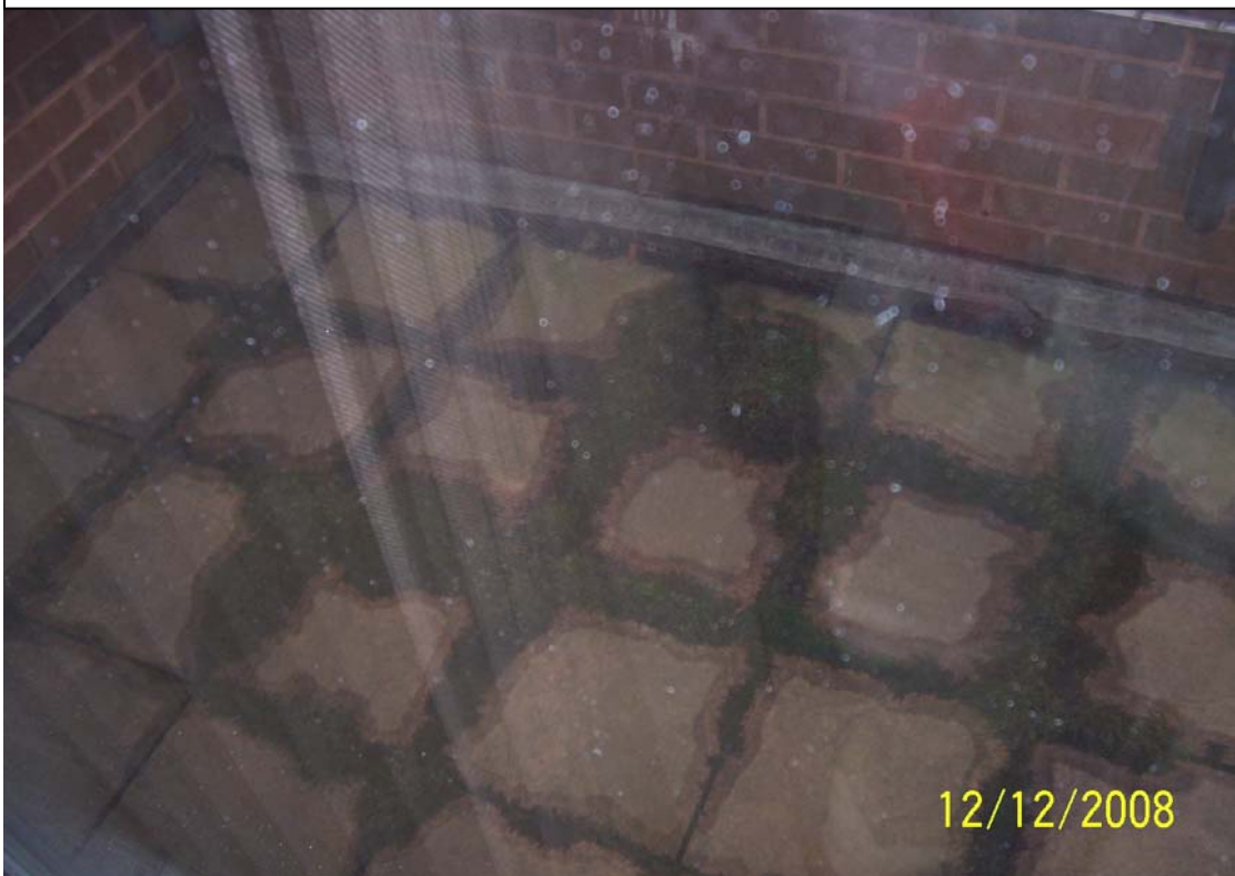
Moss Growing on Balcony on 17 th Floor
