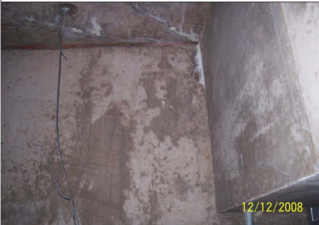
Cracks in Concrete Slab (Water leaks though cracks after in penetrated through the roof membrane)
