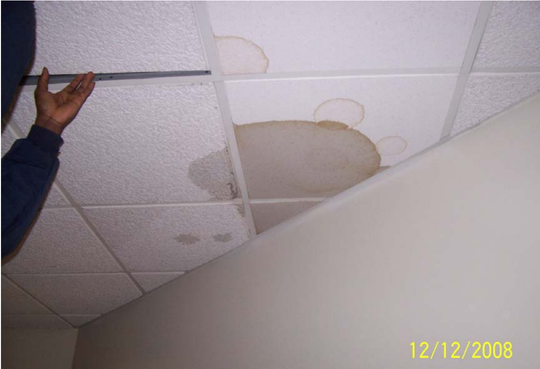
Water Damage in Conference Room on the 6 th Floor
