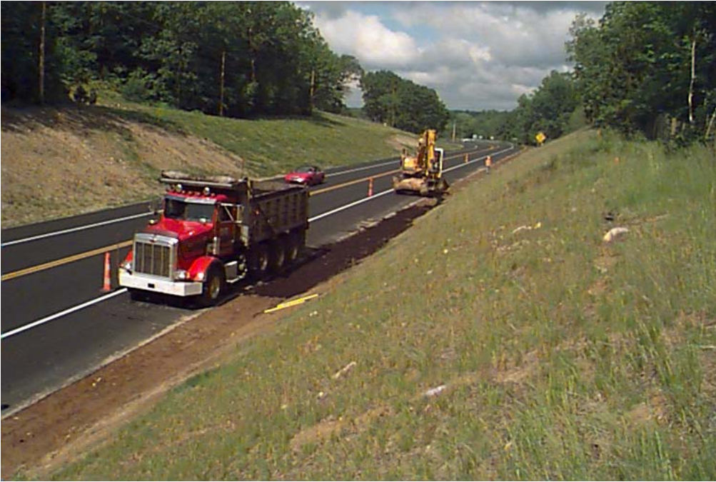
Photo #6. Placing the Compost in Sections B2 and C2 (station 266+88 – 267+88) in Drainage Swale at Bottom of Slope
