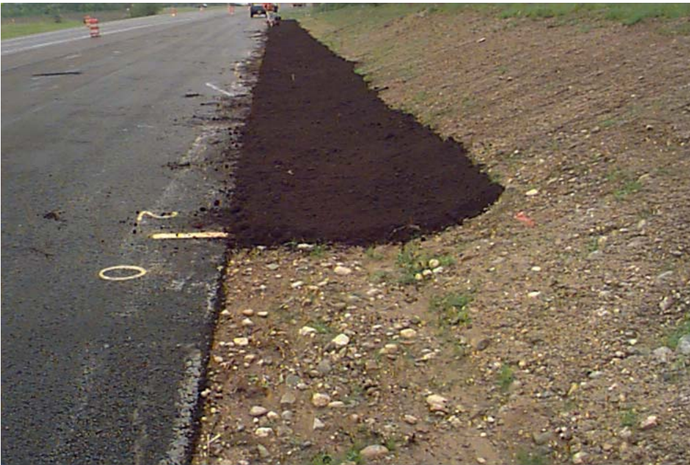
Photo #1. Two-inch Layer of Compost Placed in Drainage Swale Prior to Rototilling (station 122+68)
