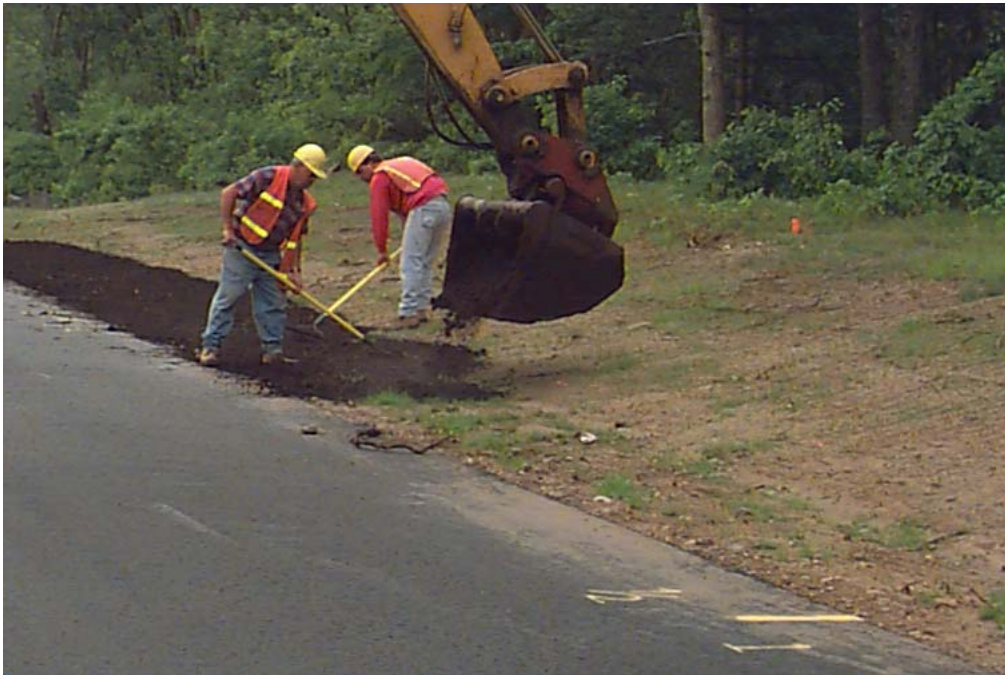
Photo #5. Placing the Compost in Section D1 (station 123+68) to ½ inch Thickness before Rototilling
