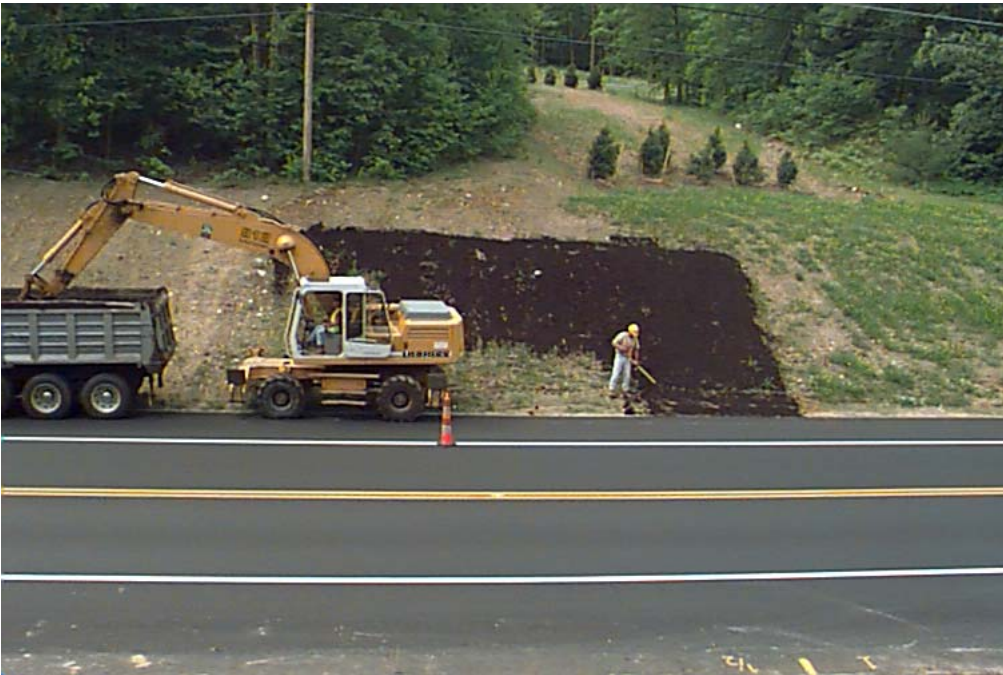
Photo #9. Station 267+50, Excess Compost Placed on 2:1 Slope (see also Photo #2)
