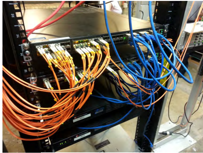
Two Cisco core switches
