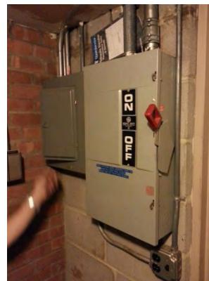
Main 200A/3P disconnect switch for elevator
