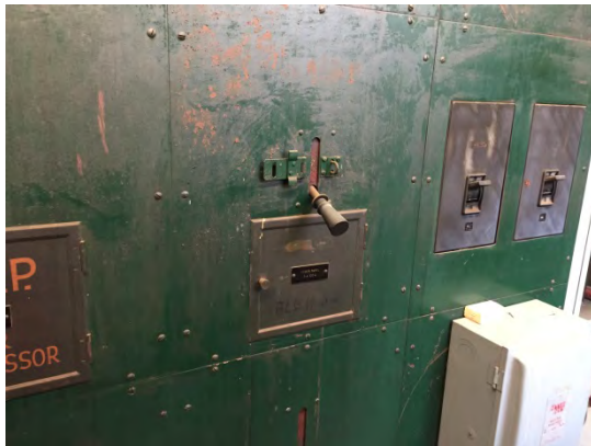
100A fused switch feeding building #52 (located in building #6)
