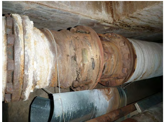
Existing Leaking Expansion Joint
