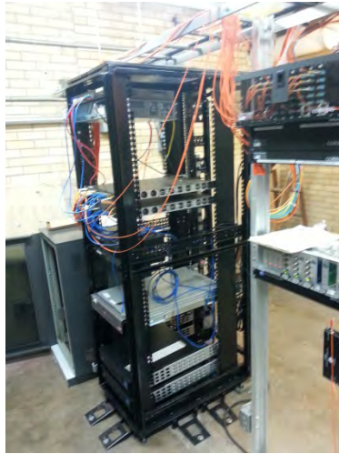
Head-end rack in basement of building #5
