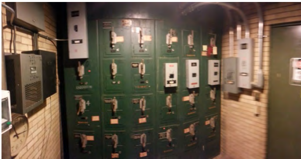
East switchgear (800A/3P)
