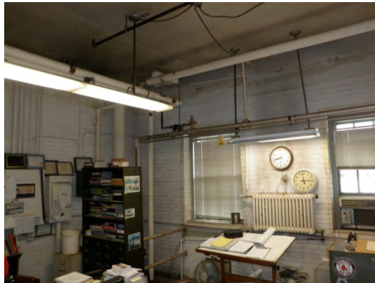
Typical T8 fluorescent fixtures
