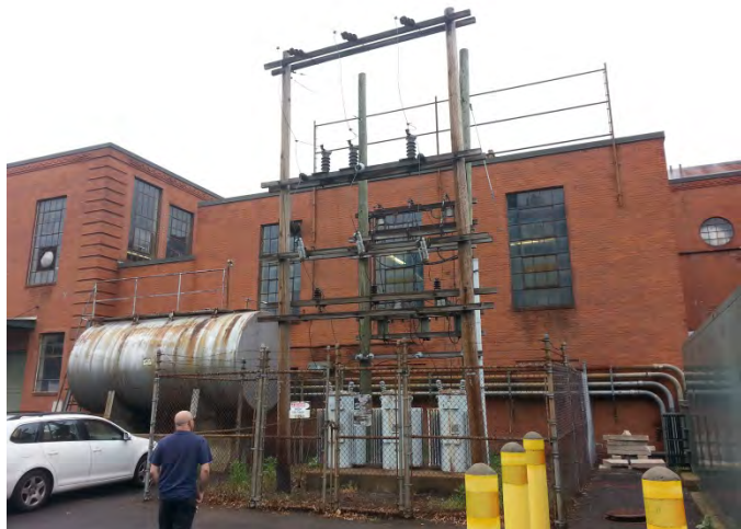
(3) 333kVA 24kV-2.4kV transformers
