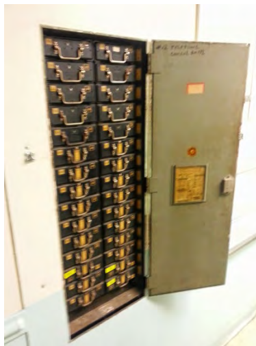
Typical fuse box
