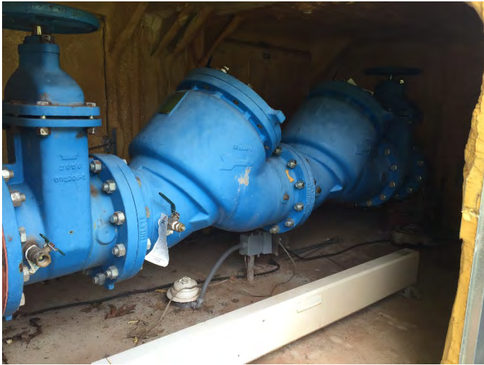
Incoming Water Service through "Hot Box"
