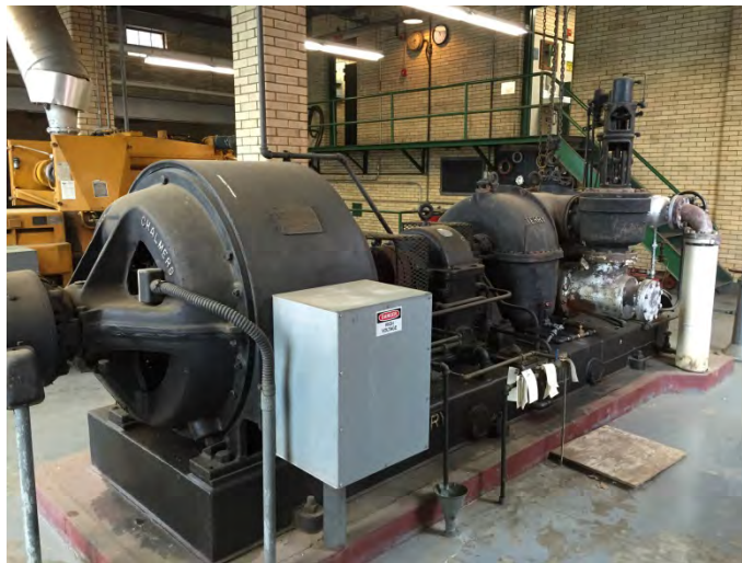
250KW, 3Ø Steam Generator
