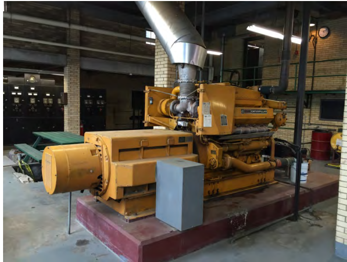
500KW, 3Ø Diesel Generator
