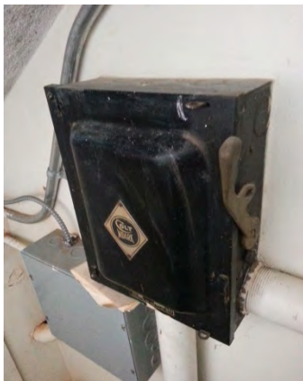
100A/3P main switch
