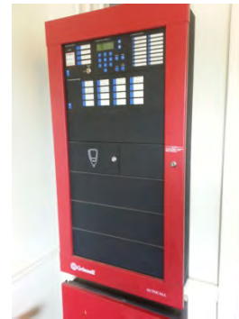
Fire alarm control panel
