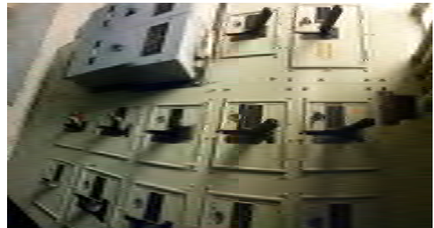
West switchgear (800A/3P)
