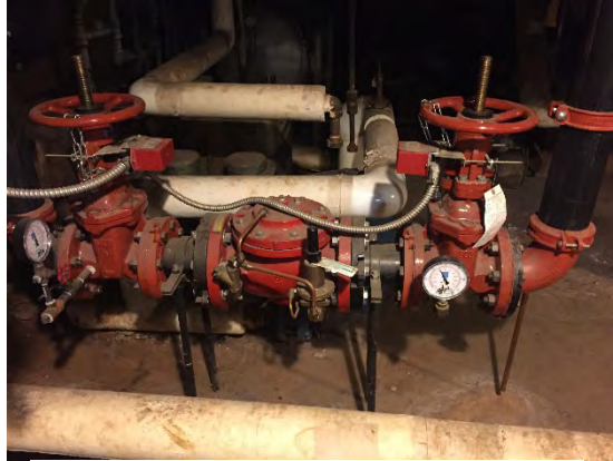
Fire Protection check valve assembly
