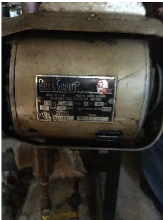
Hot Water Pump
