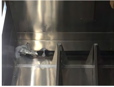
Freezing Pipe in Walk-in Cooler
