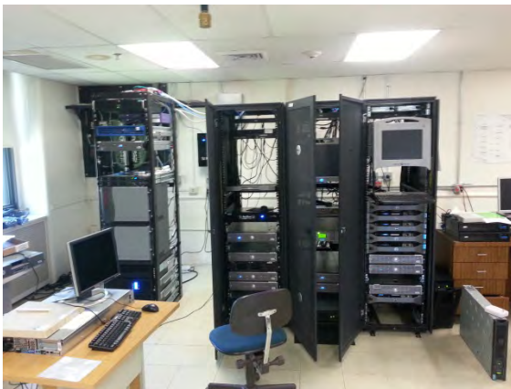
Server racks on third floor
