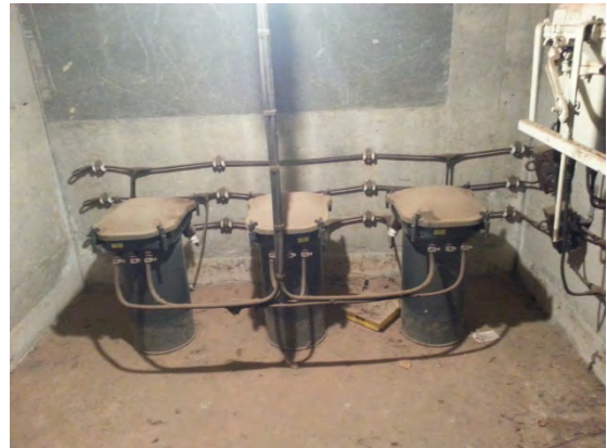
Three 45KVA transformers
