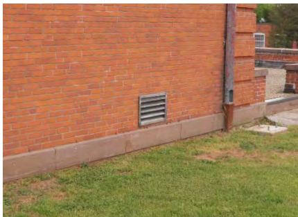
Auditorium Ventilation Louver
