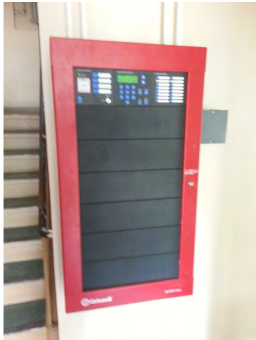
Autocall fire alarm control panel
