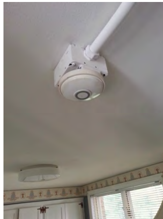
Heat detectors in the kitchen
