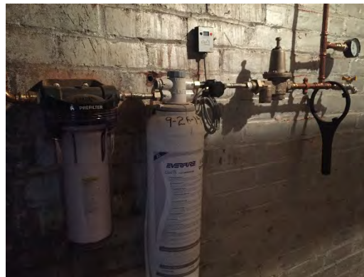
Domestic Water Filtration System
