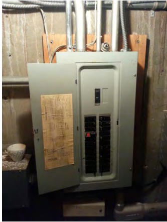
Typical MCB load center
