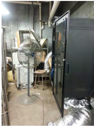
I.T. rack with no ventilation
