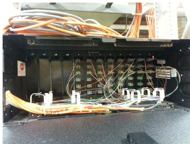
4U patch panel distributing fiber to campus
