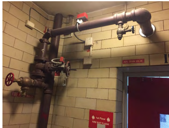
Standpipe Assembly in Stairwell
