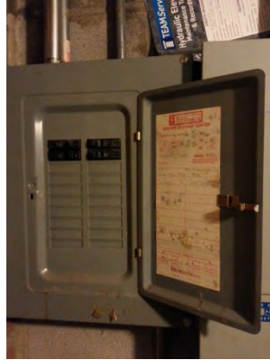
Typical branch load center
