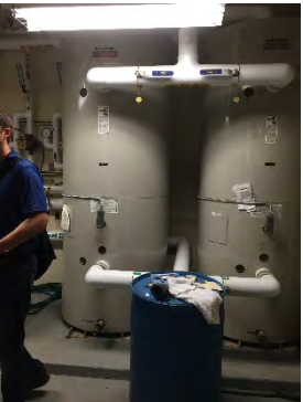
Domestic hot water storage tanks
