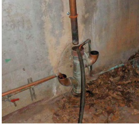
Domestic water for cooling discharges to sewer
