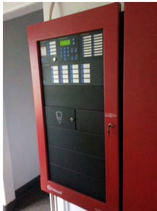
Simplex fire alarm control panel
