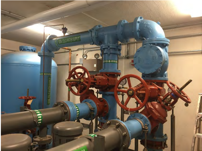
Domestic Water System
