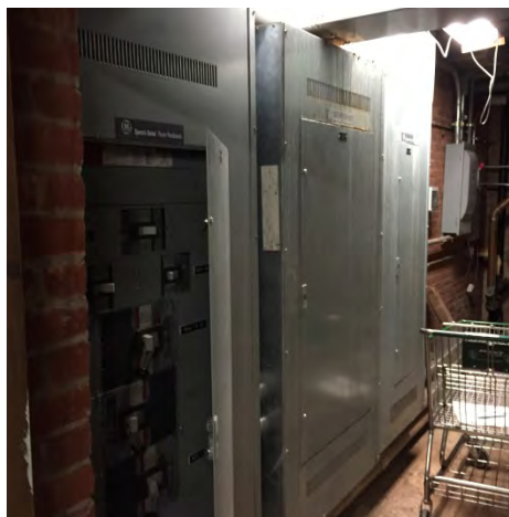
Two-Section Main distribution switchboard
