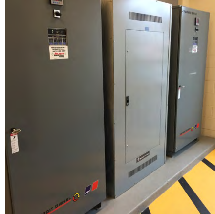
Critical power and life safety ATS's
