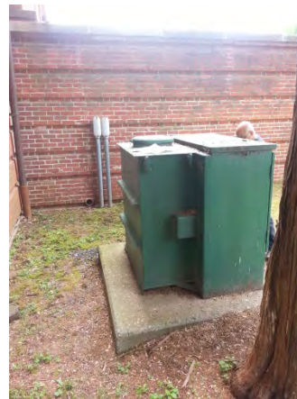
Exterior 112.5KVA transformer
