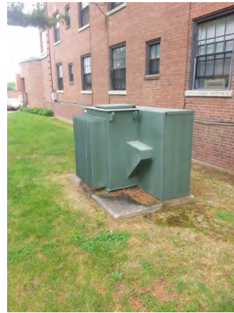
Exterior 225KVA transformer
