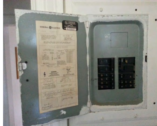
Typical recessed branch panel
