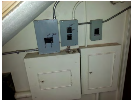
Distribution gear located under the main staircase
