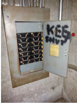
Main distribution fuse box
