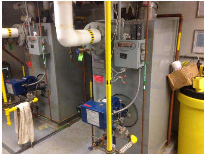
Hot Water Boilers
