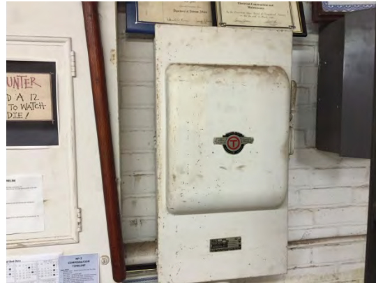
200A main disconnect switch in building #52
