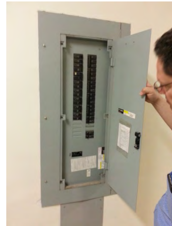
Newer panelboard for HVAC expansion
