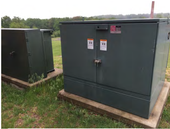
MTS (right) and transformer (left)
