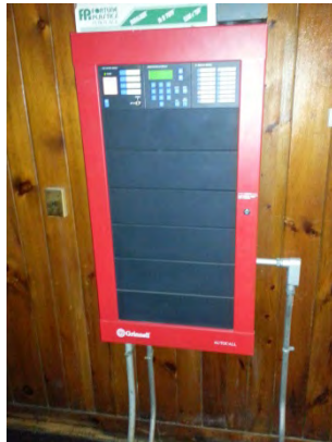
Fire alarm control panel located in main corridor
