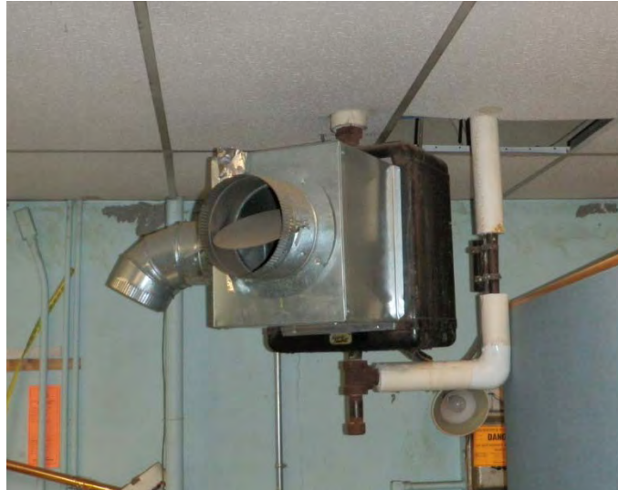
Steam Unit Heater
