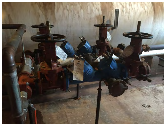
Domestic water system
