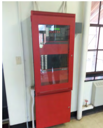
Simplex control panel
