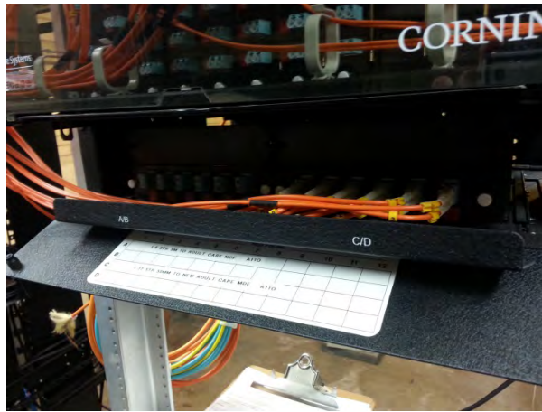
Fiber strands in building #5 feeding the ACF
