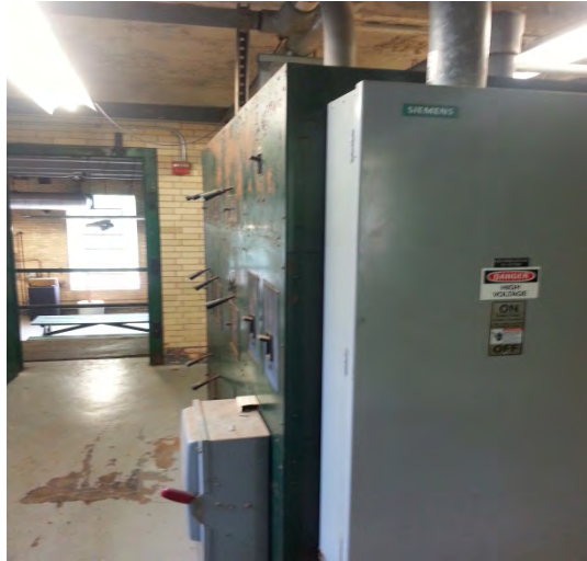
Main 600A/3P fused switch and distribution switchboard
