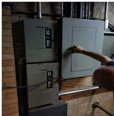
Main 200A/3P disconnect switch and distribution panel
