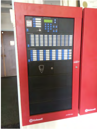
The building's FACP is not operational
