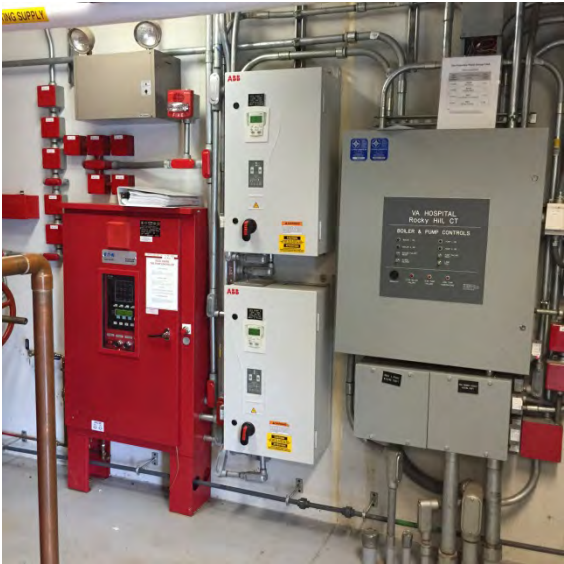
Fire pump controller and VFD's for hot water circulation pumps
