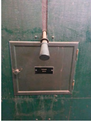
200A fused switch feeding building #8
