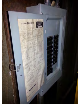
Typical MLO load center
