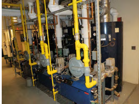
Hot Water Boilers
