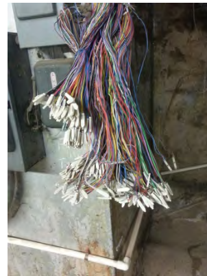
Phone wiring splicing
