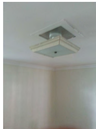
Lighting fixture NOT original to building
