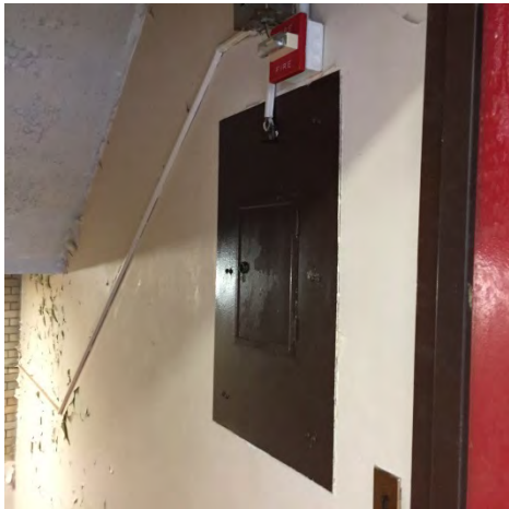
Older fuse-box style panel, located in stairwell
