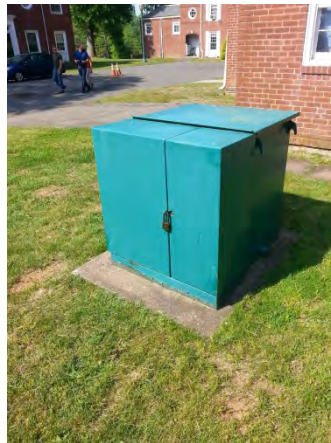
Exterior transfer switch / transformer
