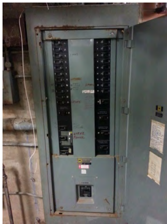
Main distribution panel in basement (with 400A MCB)
