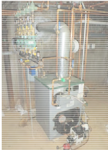
Typical HW Boiler
