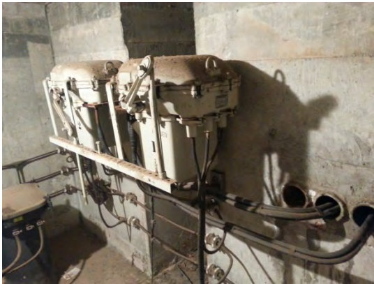
Two high-voltage circuit breakers
