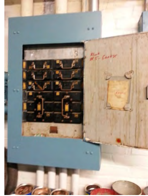
Main distribution fuse box in building #8
