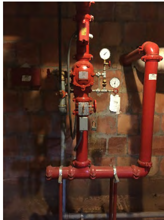
Fire Protection Riser
