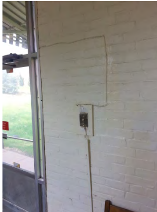
Ethernet jack with exposed wiring
