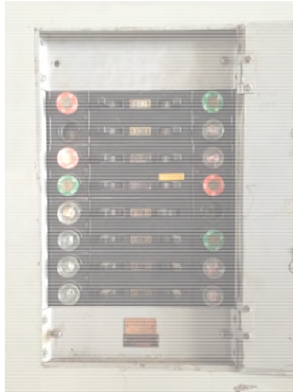
Typical fuse box
