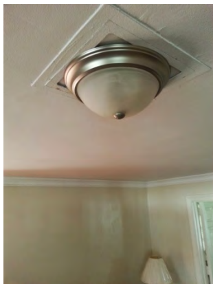
Lighting fixture NOT original to building
