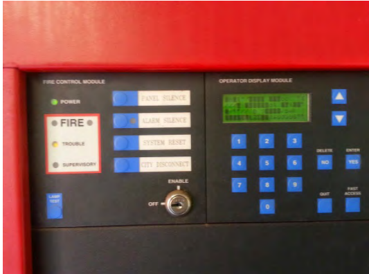
FACP is not operational.
