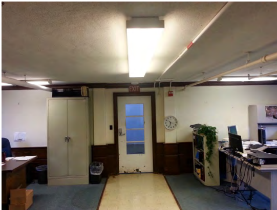
Typical fluorescent lighting
