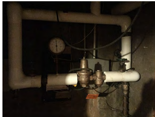
Domestic water feed into basement
