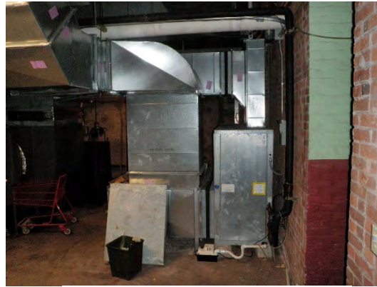
Auditorium Split System
