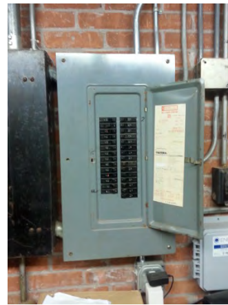
Typical branch panel (load center)
