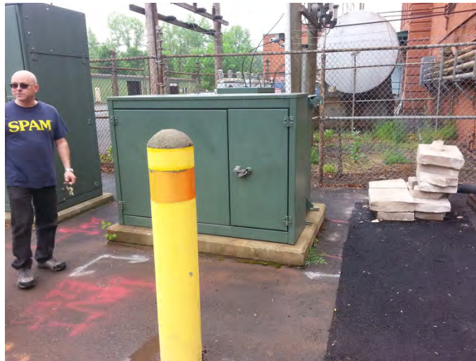
225KVA, 24kV-208V transformer
