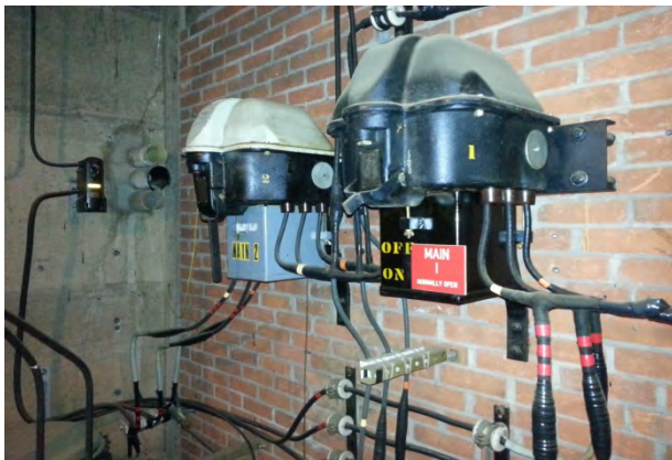
Two high-voltage circuit breakers
