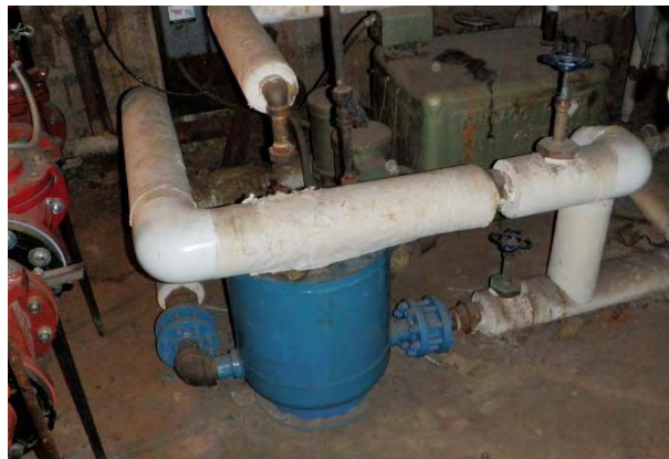
Steam driven condensate pump
