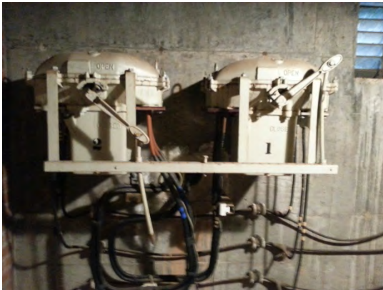
Two high-voltage circuit breakers
