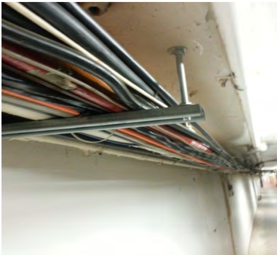
Cabling in tunnels
