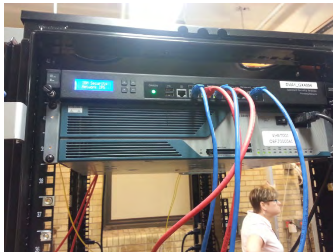
Main campus firewall (Top) and router (bottom)
