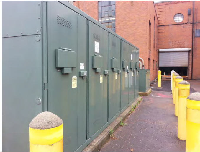
Campus distribution switchgear
