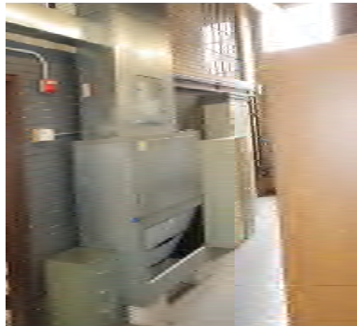
DX Cooling Unit in Warehouse
