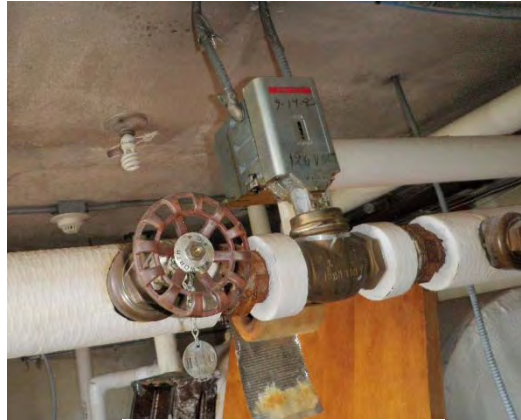
Steam Control Valve
