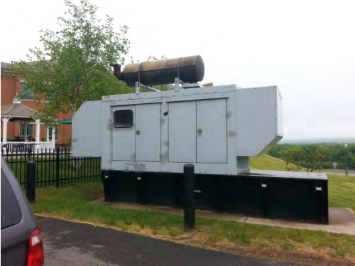
300KW diesel generator
