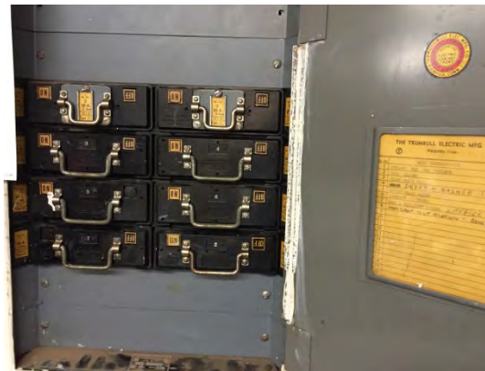
Main fuse box
