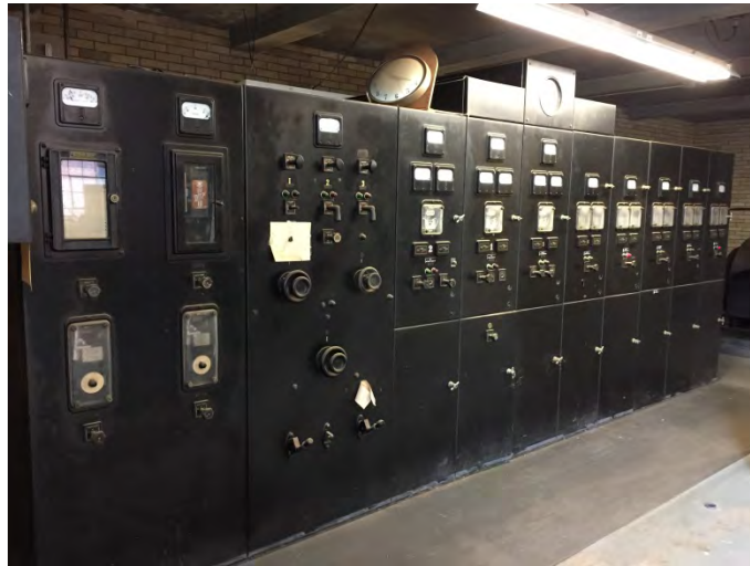
The campus’ original high-voltage switchgear
