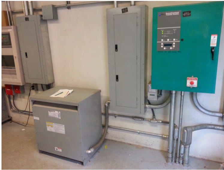
From left to right: 208V distribution panel, 45KVA TX, 480V distribution panel, 225A/3P ATS
