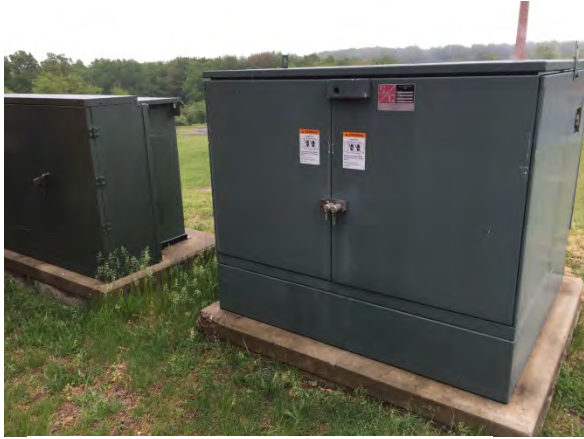
MTS (right) and transformer (left)
