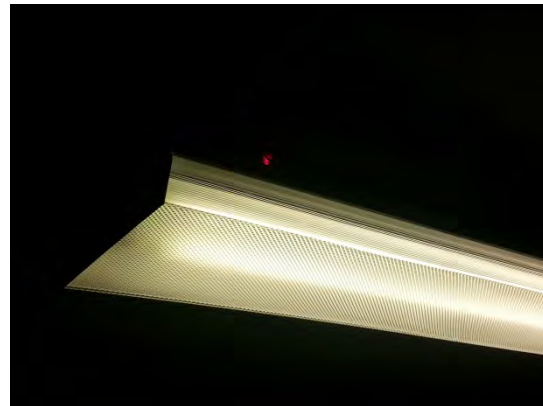
Fixture outfitted with emergency ballast
