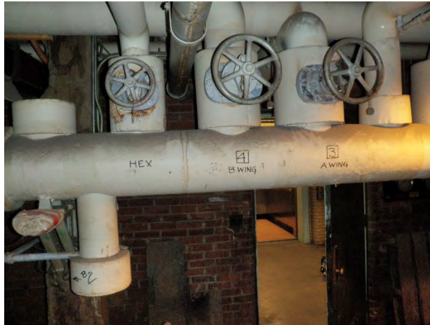
Steam valves for each wing
