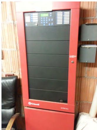
Autocall fire alarm control panel in main lobby
