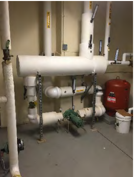
Hot water heat exchanger
