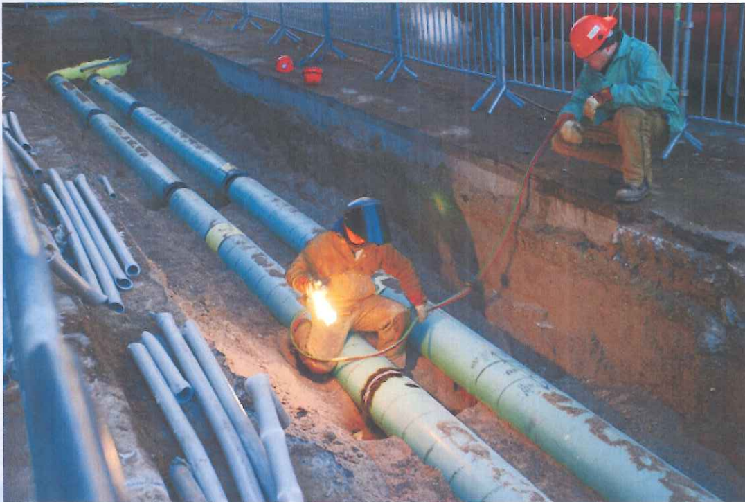
Project contractors install District Energy chilled water pipes in St. Paul, MN in February 2010
