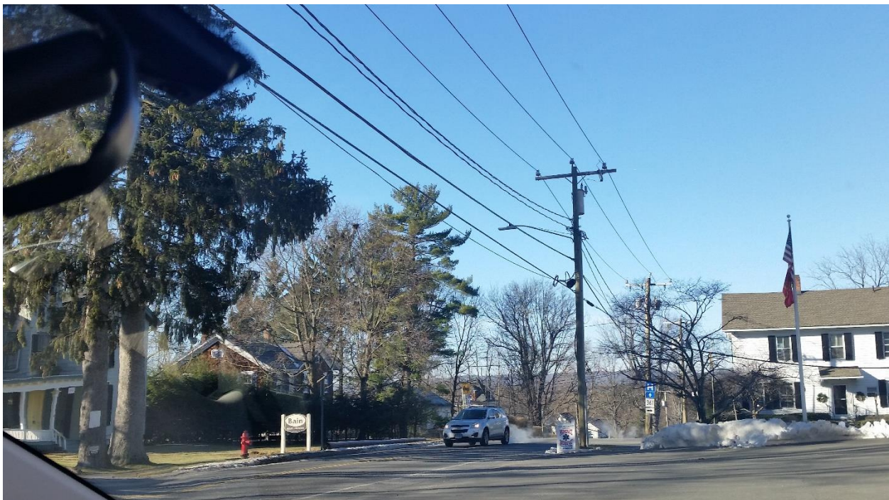
Figure 10: Sharon Hospital – Lighttower Cable and Splice Enclosure
