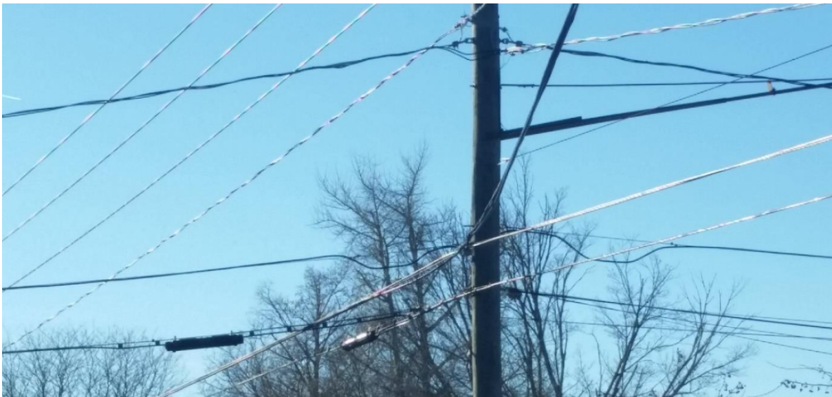
Figure 12: Congested Utility Pole in Sharon with Boxing on Both Sides of Pole
