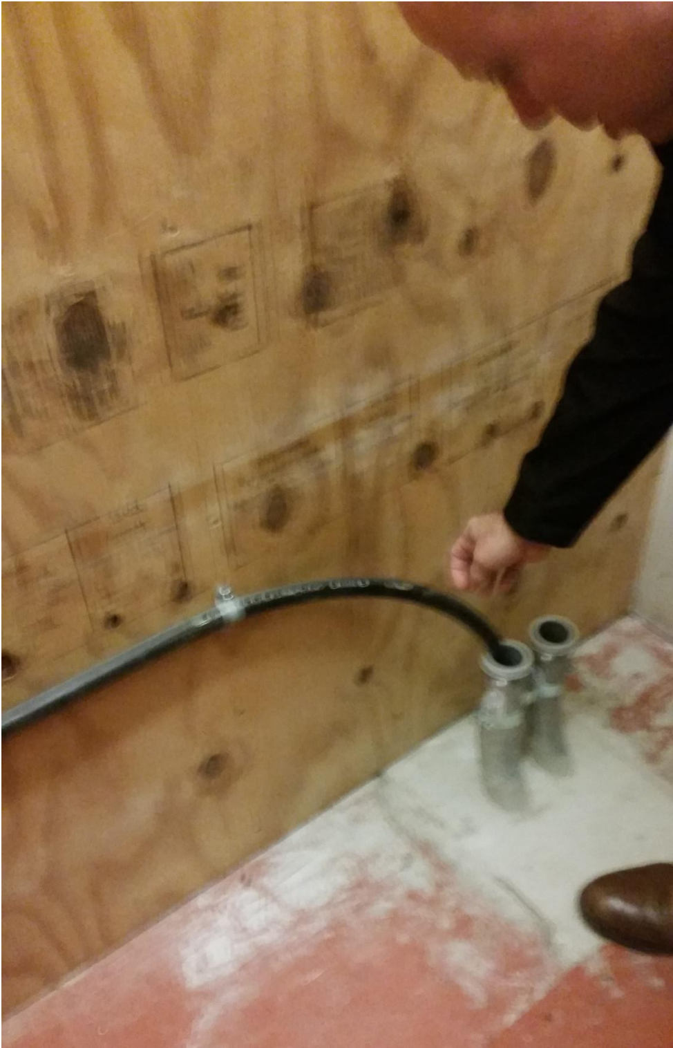
Figure 3: Conference of Churches – Conduit to Street from Inside Facility
