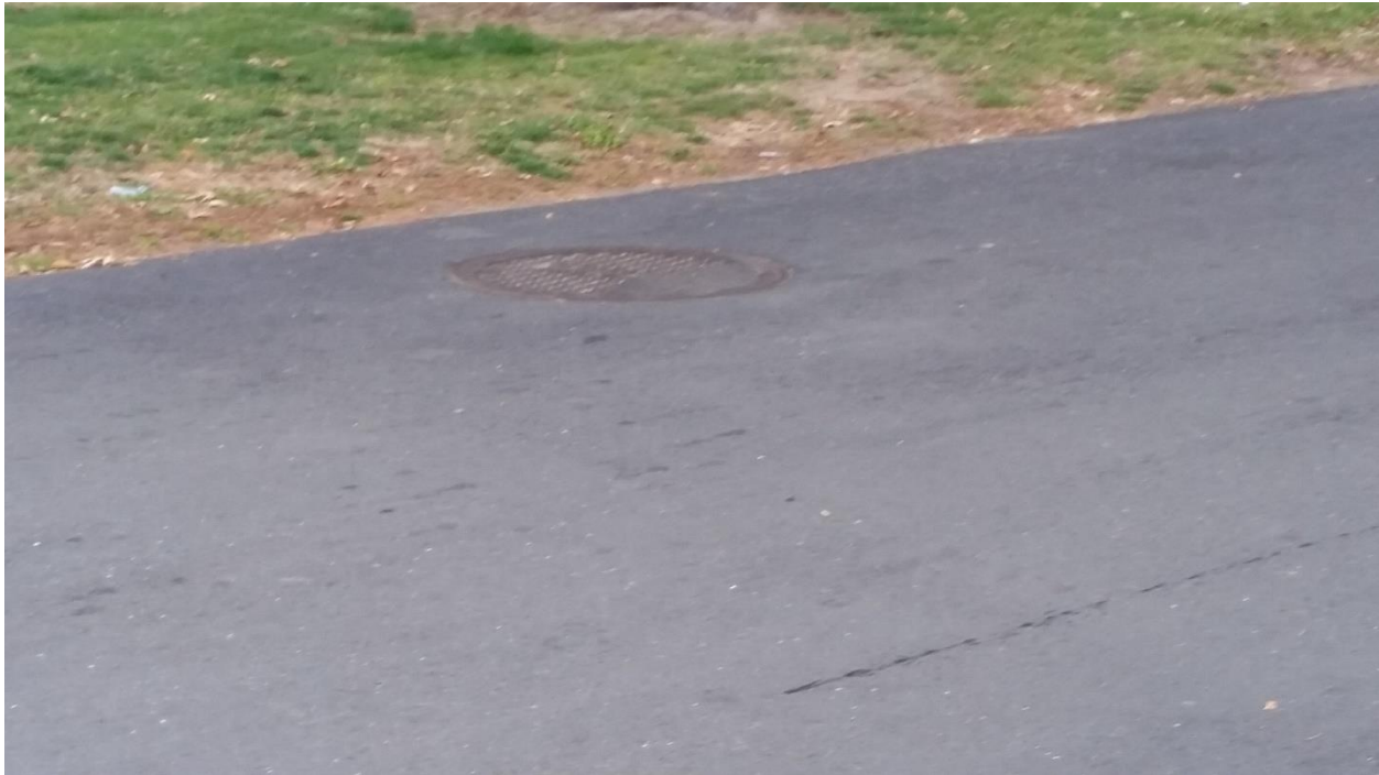
Figure 4: Conference of Churches – Manhole Where Conduit Terminates at Side of Street
