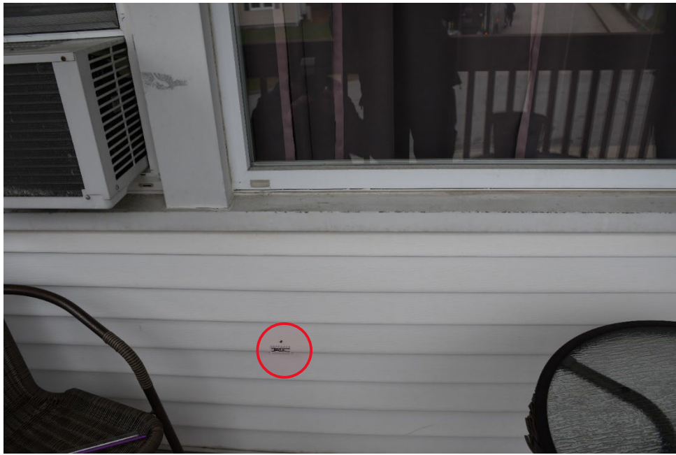
[Damage outside residence of 26 Elizabeth Street Extension]
