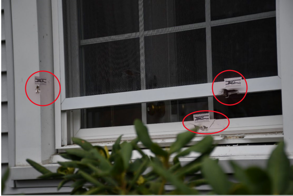
[Damage outside residence of 179 Dunham Street]
