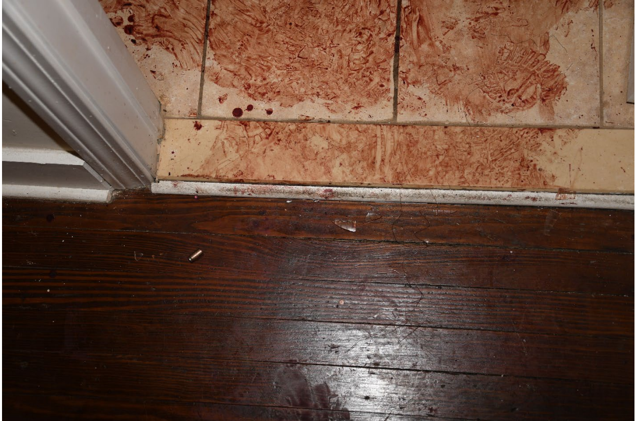
Third Floor Bathroom Threshold
