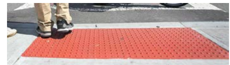
Figure 23. Tactile Warning Strip
