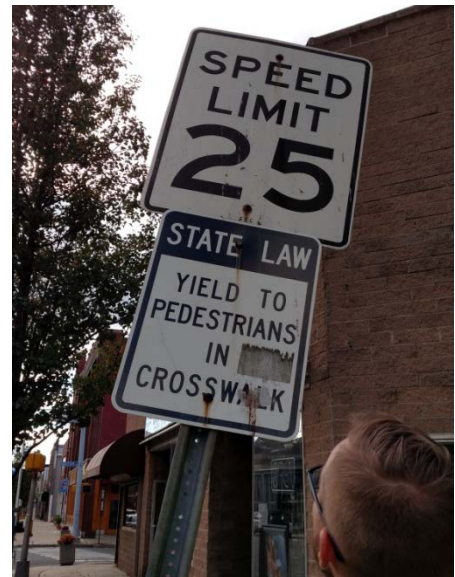
Figure 15. Sign Does Not Meet Height Requirements
