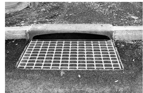
Figure 24. Bike Friendly Catch Basin Grate
