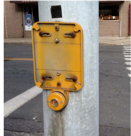
Figure 8. Push Button Missing Placard
