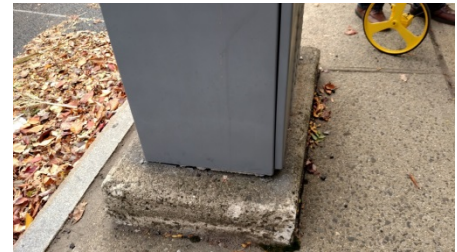
Figure 9. Rusted Traffic Control Box
