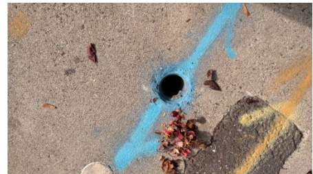
Figure 14. Handhole Missing Cover
