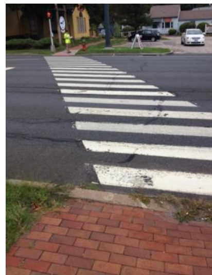
Figure 35. Angled cross on East Main Street west of Towpath Lane with no detectable warning strip on south side
