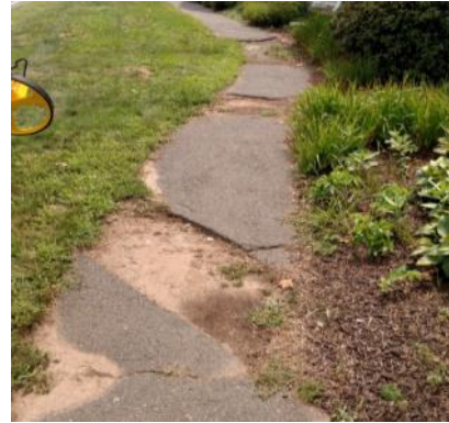
Figure 33. Broken sidewalk at Avon Village East
