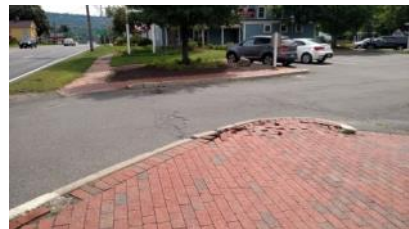
Figure 34. Missing Ramps at Old Avon Village
