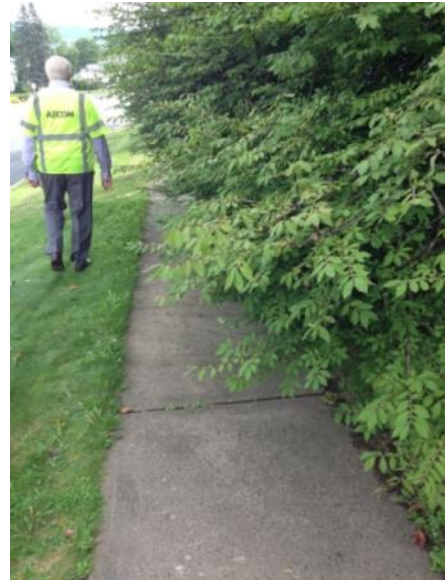
Figure 30. Overgrown vegetation on sidewalk on south side of Rt. 44 east of Ensign Drive
