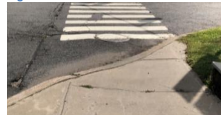
Figure 32. Lack of detectable warning strips
