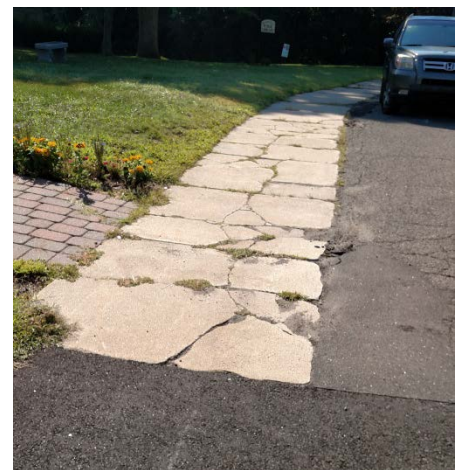
Figure 7. Broken Sidewalk in Front of Town Hall
