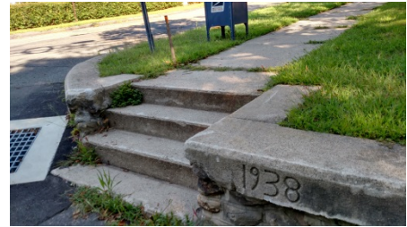
Figure 8. Stairs on Maple Street Sidewalk
