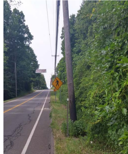
Figure 8. Utility Poles Close in on Roadway
