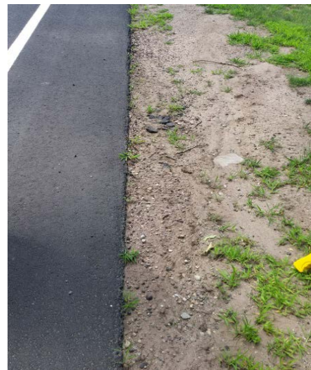
Figure 8. Drainage Issue on Notch Road
