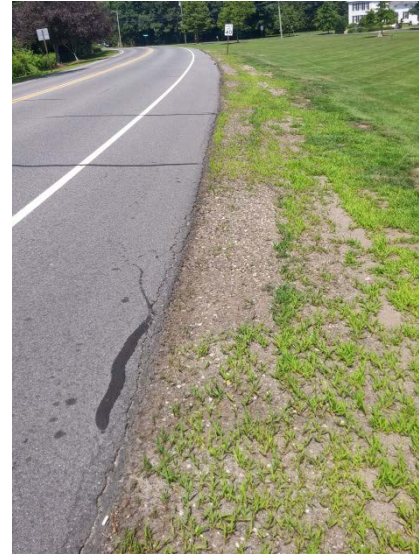
Figure 12. Drainage Issues by Library Green
