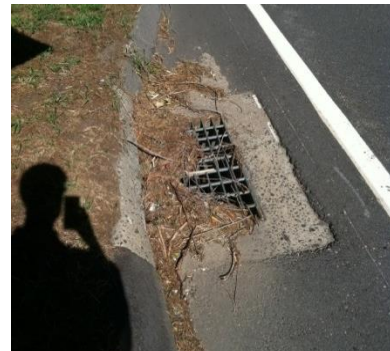
Figure 10. Debris in Catch Basin Grate
