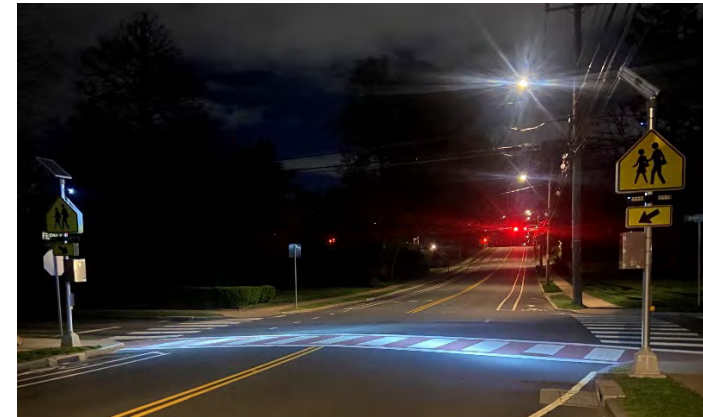
Exhibit 42: An example of a crosswalk high intensity light integrated with an RRFB at night in West Hartford, CT. Note – The yellow flashers are not activated in this photo to demonstrate the crosswalk light.
