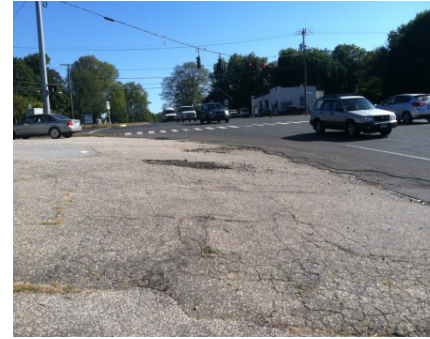
Figure 7. Poor Access Control at Northwest Corner of Routes 87 and 66 Intersection
