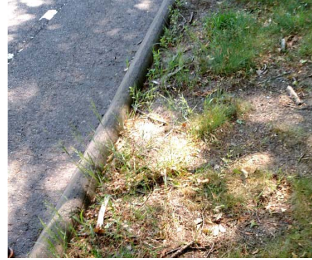
Figure 13. Soil Below Curb Line
