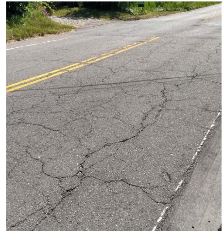
Figure 5. Poor Roadway Condition on Route 31
