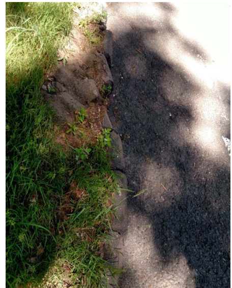
Figure 12. Broken Curbing at Winterberry Lane
