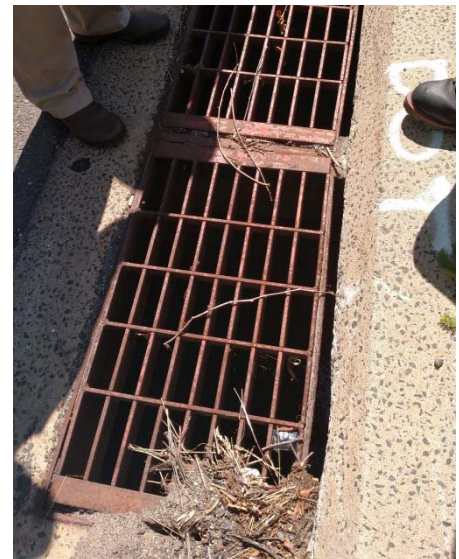
Figure 6. Non-bicycle Friendly Catch Basin Grates
