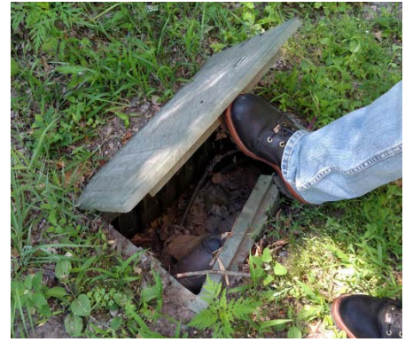
Figure 16. Broken Hand Hole
