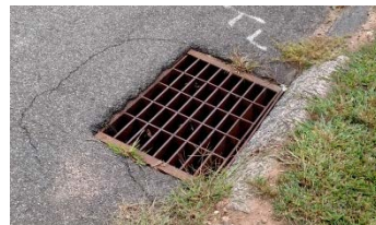
Figure 14. Non-bicycle friendly catch basin grate
