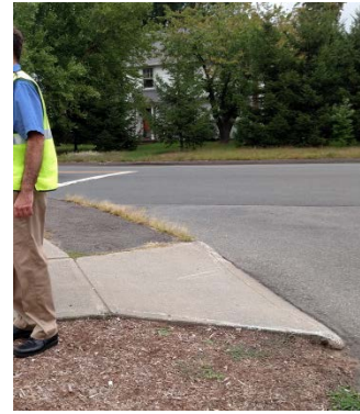
Figure 16. No tactile warning strip on ramp
