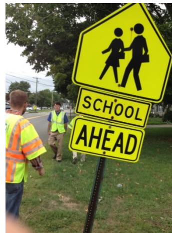
Figure 18. Tilted school crossing ahead sign on westbound Court Street west of Court Place
