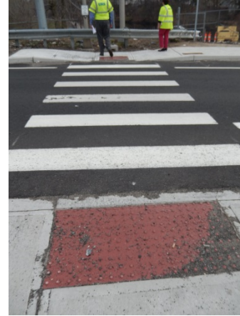
Figure 14: Pedestrian button location is not accessible
