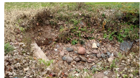
Figure 11. Culvert Which is Easily Clogged
