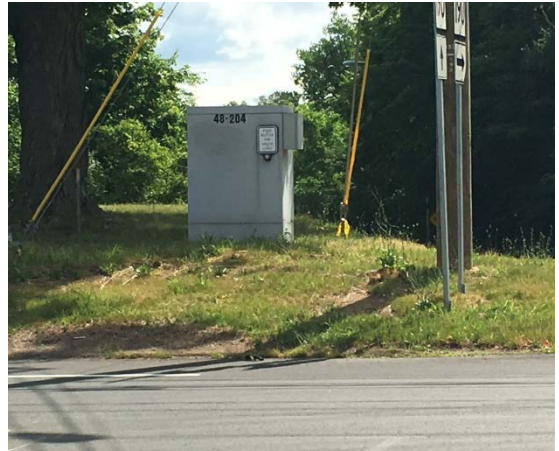
Figure 11. Pushbutton Located on Utility Box
