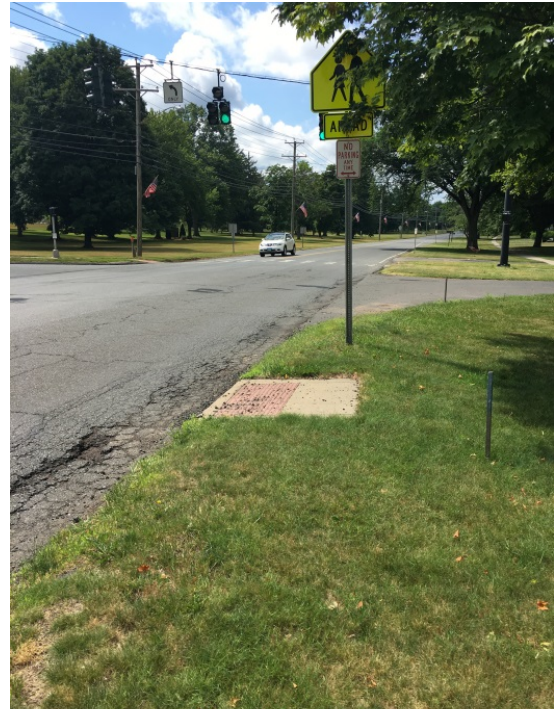
Figure 8. Ramp Not Connected to Sidewalk
