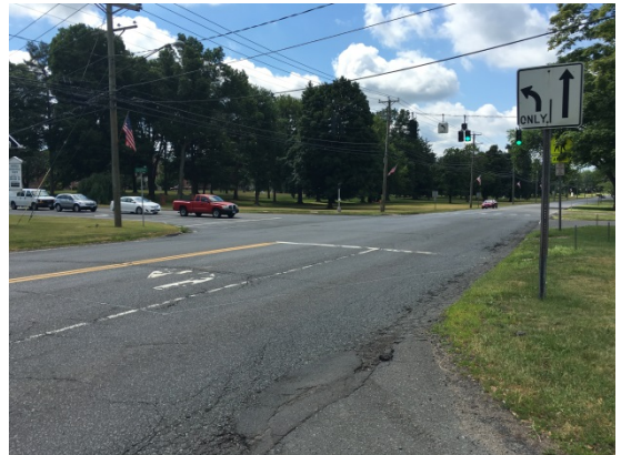
Figure 12. Shoulder Area is Not Defined by Striping
