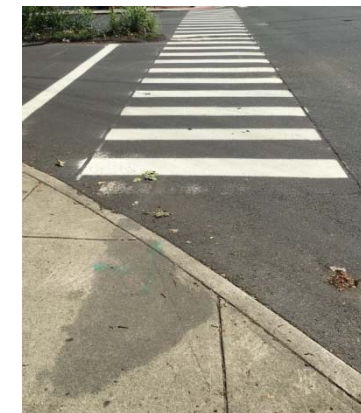
Figure 10. Missing pedestrian push button and detectable warning strip
