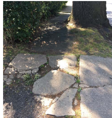
Figure 13. Poor sidewalk condition
