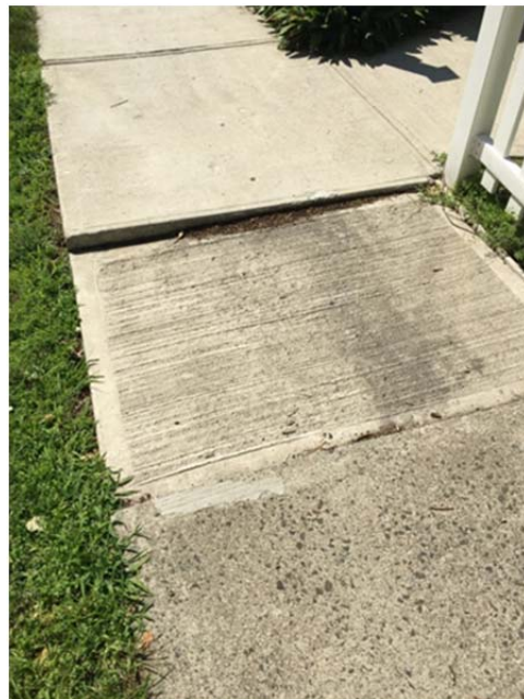
Figure 19. Repair uneven sidewalk
