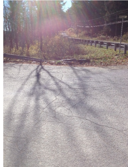
Figure 13: Damaged guardrail on southeast corner of White's Woods Road and Webster Road
